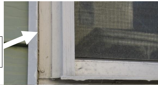
Missing window sill horn
