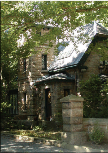
A regular maintenance program has kept this unique stone home in top shape though the years. Inspect regularly for cracks, settlement, vegetation, moisture damage, deteriorating mortar, and loose or missing masonry units.
