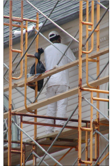
Paint should be removed from surfaces in the gentlest means possible to avoid damaging the historic material. Several stories above the ground, this man carefully removes paint from the exterior of Trinity Church by hand scraping.
