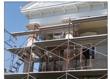
Paint removal in progress at a home on Historic Hill. Only remove paint until you come to the first sound layer. Avoid taking off too many layers. Stripping a feature to bare wood destroys its record of historical paint schemes.
