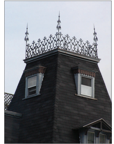
Metal cresting atop a tower on a Second Empire style home. Such architectural elements can be hard to get to for inspection, but features such as this are crucial to defining a building's individual character.
