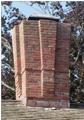
It is also important to maintain your chimneys. Chimneys are often prominent features of historic homes in Newport, and great care should be taken to ensure they last for hundreds more years. This unique chimney is on a colonial-era home located on The Point.
