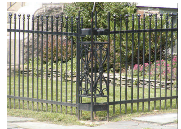
It is important to maintain a sound paint film on features such as cast-iron gates and fences in order to prevent corrosion. Cast iron fences are common in many of Newport's historic neighborhoods.
