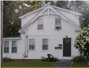
The last vestige of this modest house's former identity is found in its sole surviving wooden crossbracing. The rest of the decorative elements that this house may have once had have been removed, probably because the vinyl siding could not fit such details. There is a chance, however, that wooden clapboards still exist underneath the vinyl; and example of this was shown in the section on Wood.
