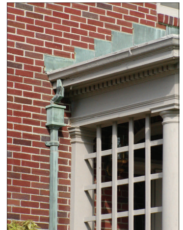
Some metals are both decorative and functional, such as this copper flashing and downspout. Copper develops a distinctive patina with age which is prized for its beauty, and should not be disturbed.
