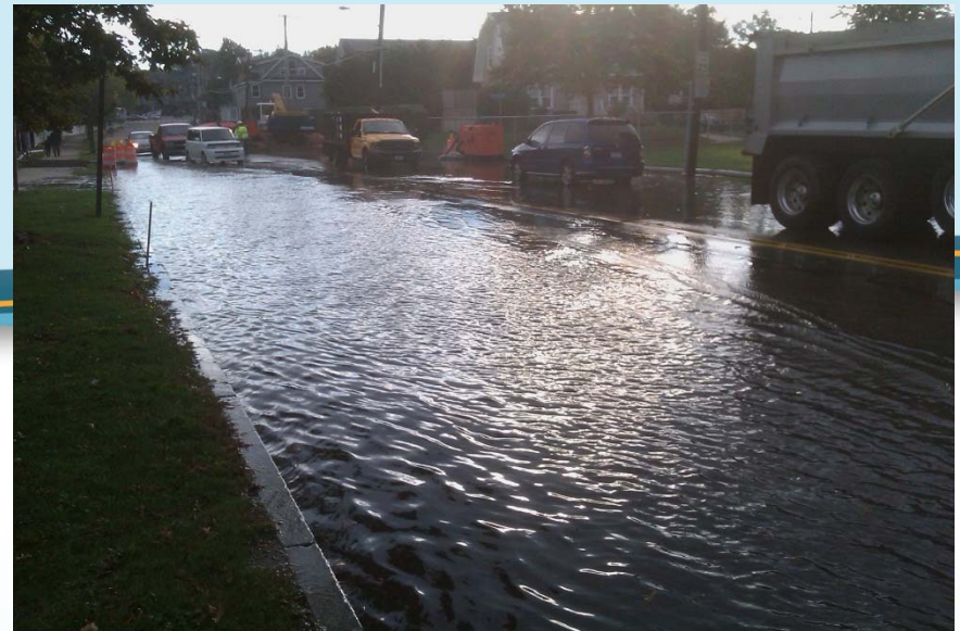
Tidal flooding at Wellington Avenue in 2011
