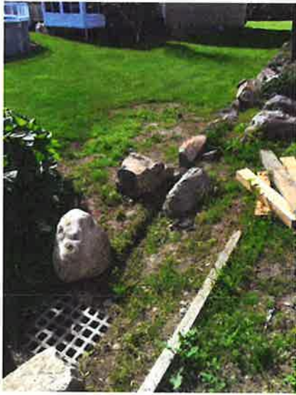
Figure 10. Catch Basin behind 29 Wilbur Avenue
