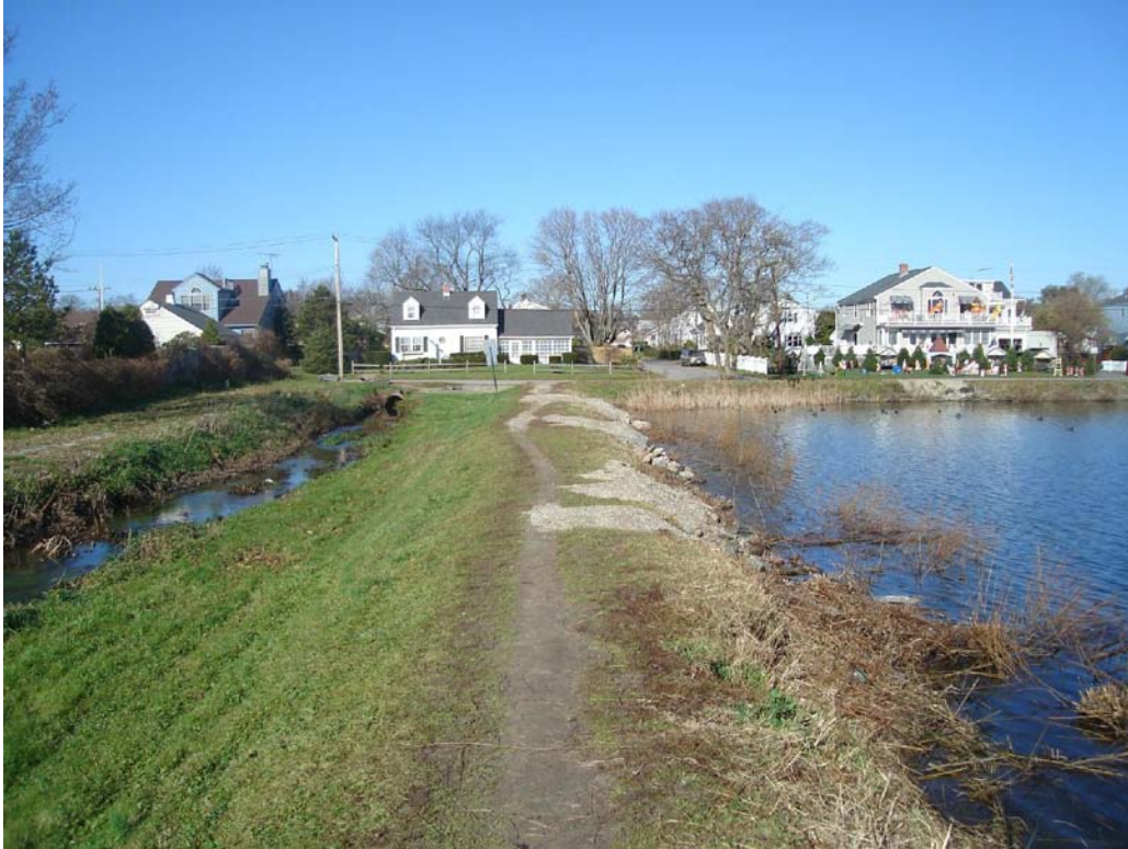
Sta. 57+57: Photo of Moat and Adjacent Pond Embankment (Looking in Upstream Direction)
