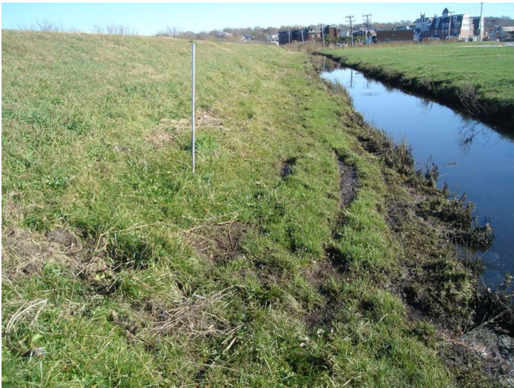
South Embankment - Wet area with rutting on narrow bench along downstream toe of slope
