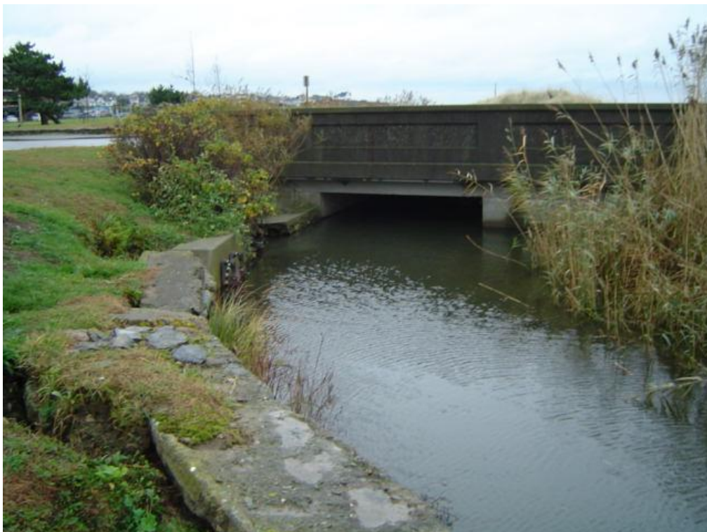
Sta. 2+97: Photo of Upstream Side of Memorial Avenue Culvert (Looking in Downstream Direction)
