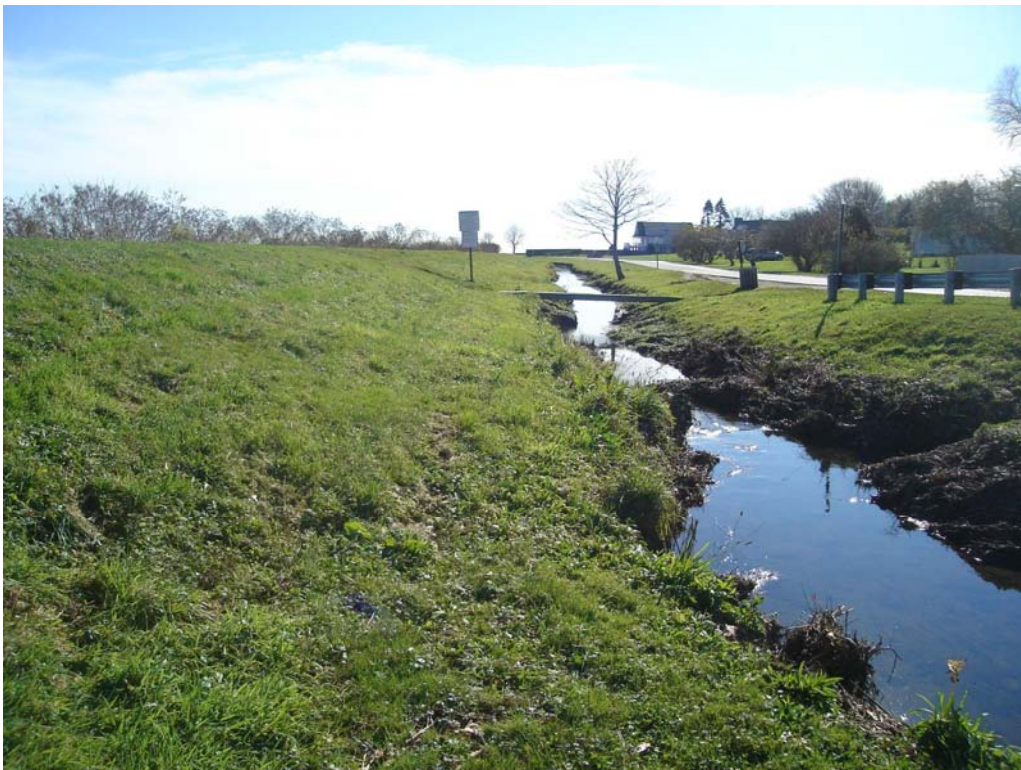
West Embankment – Narrow bench along downstream toe of slope, erosion along moat channel
