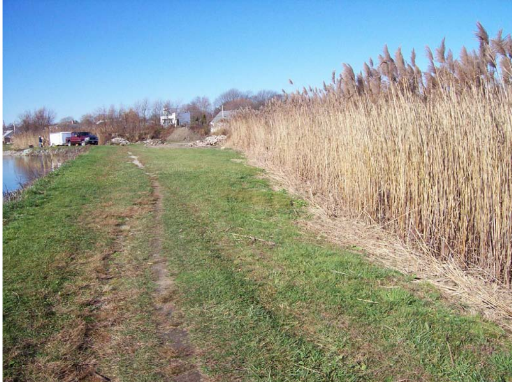
Sta. 80+58: Photo of Embankment and Low-Lying, Marsh Area (Looking in Downstream Direction)
