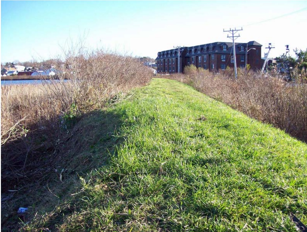
South Pond Spillway - Settlement adjacent to left spillway abutment
