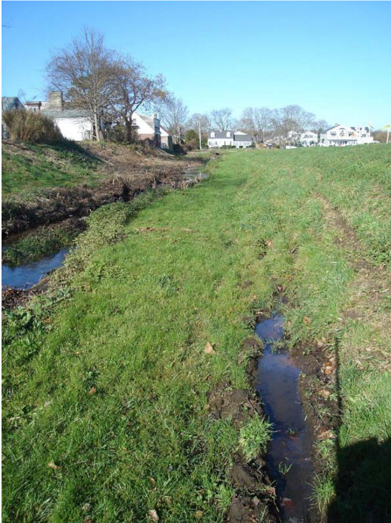
West Embankment – Saturated bench and rutting along downstream toe of slope
