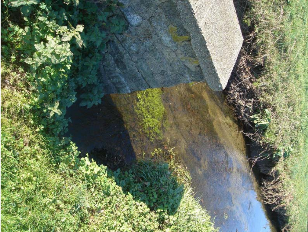
Erosion at upstream end of left wall along moat channel
