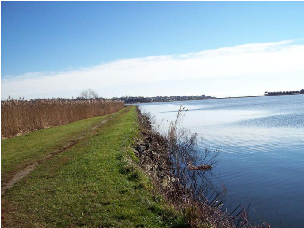
Sta. 80+58: Photo of Embankment and Low-Lying, Marsh Area (Looking in Upstream Direction)
