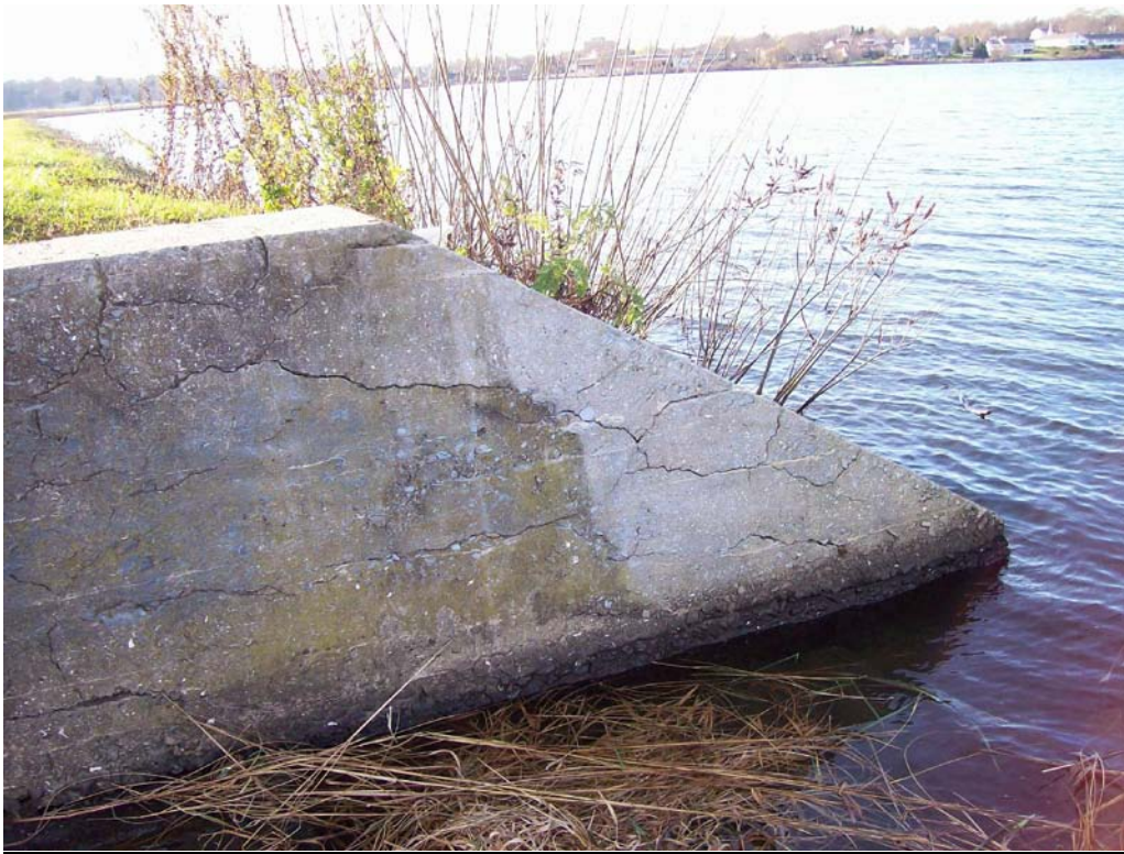
North Pond Primary Spillway - Cracking at face of right abutment
