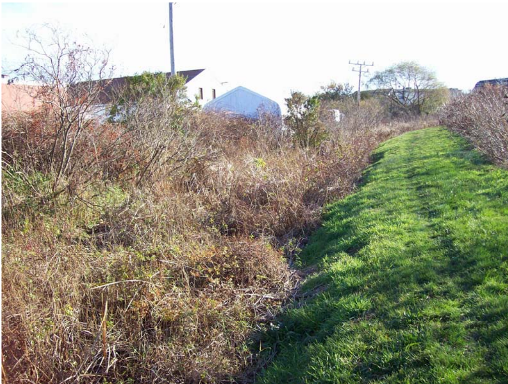
East Embankment - Vegetation on embankment, narrow crest width
