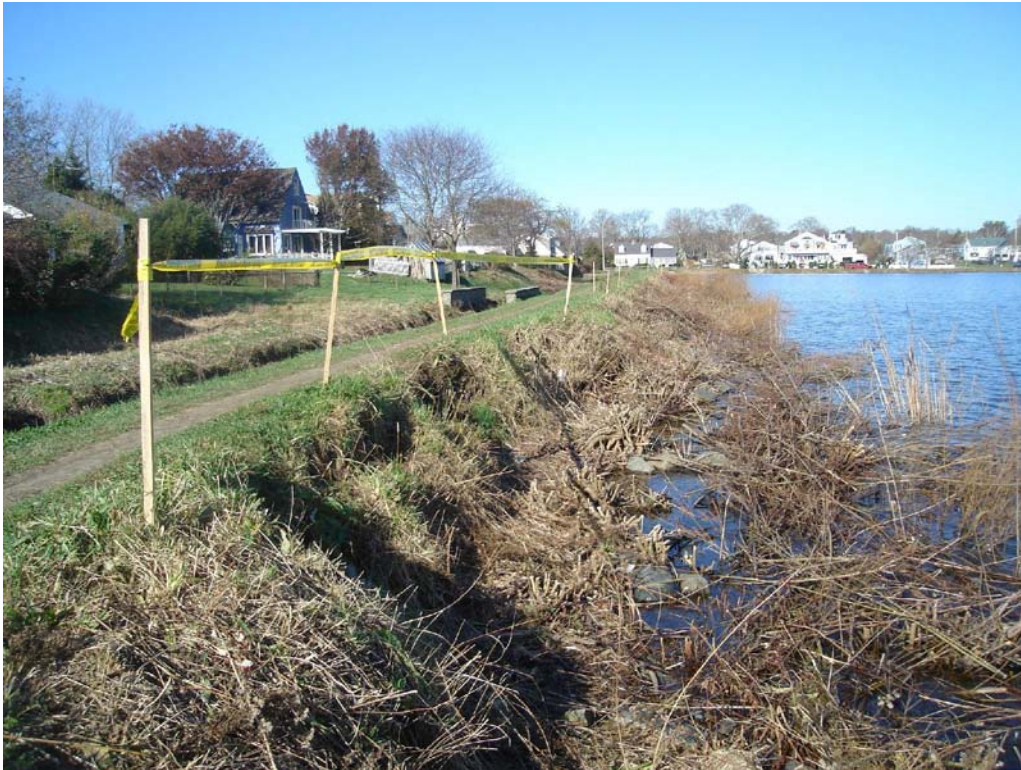
West Embankment – Severe scarps on upstream slope resulting in narrow crest width
