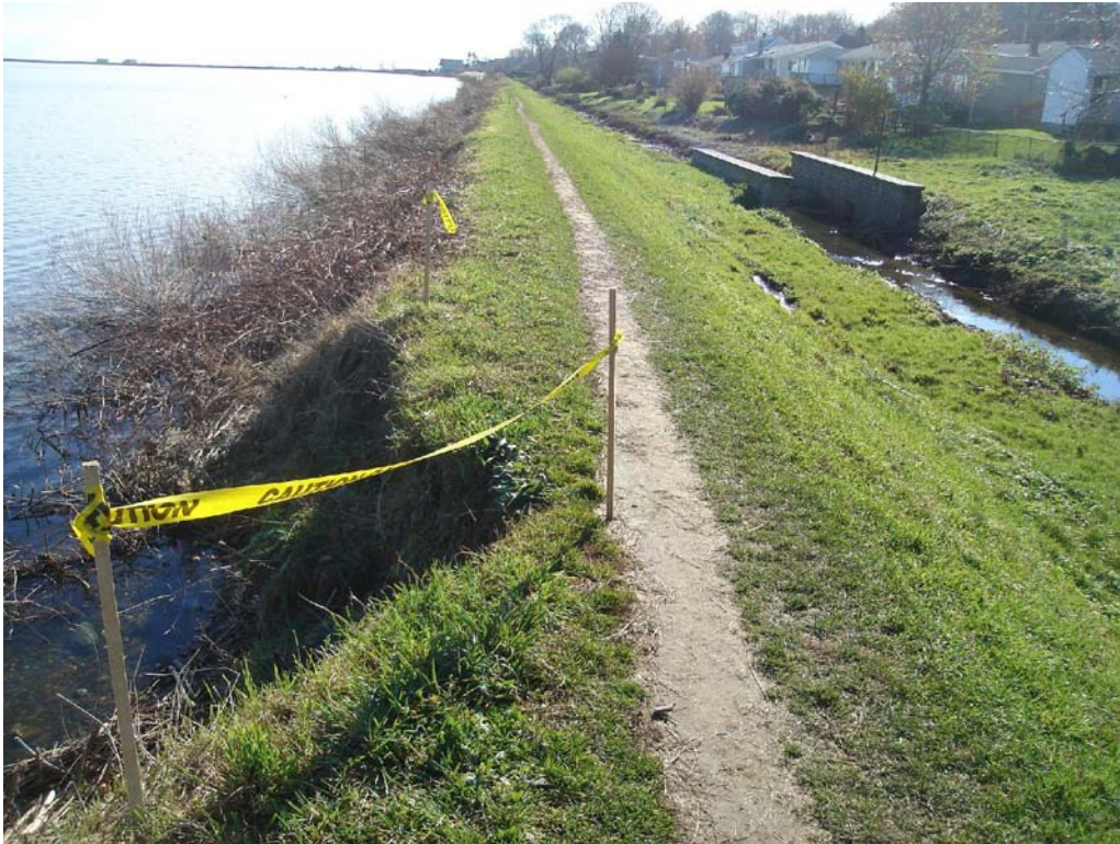
West Embankment – Severe scarp on upstream slope resulting in narrow crest width
