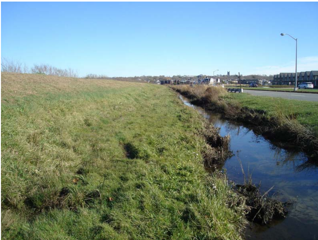
South Embankment - Wet area with rutting on narrow bench along downstream toe of slope
