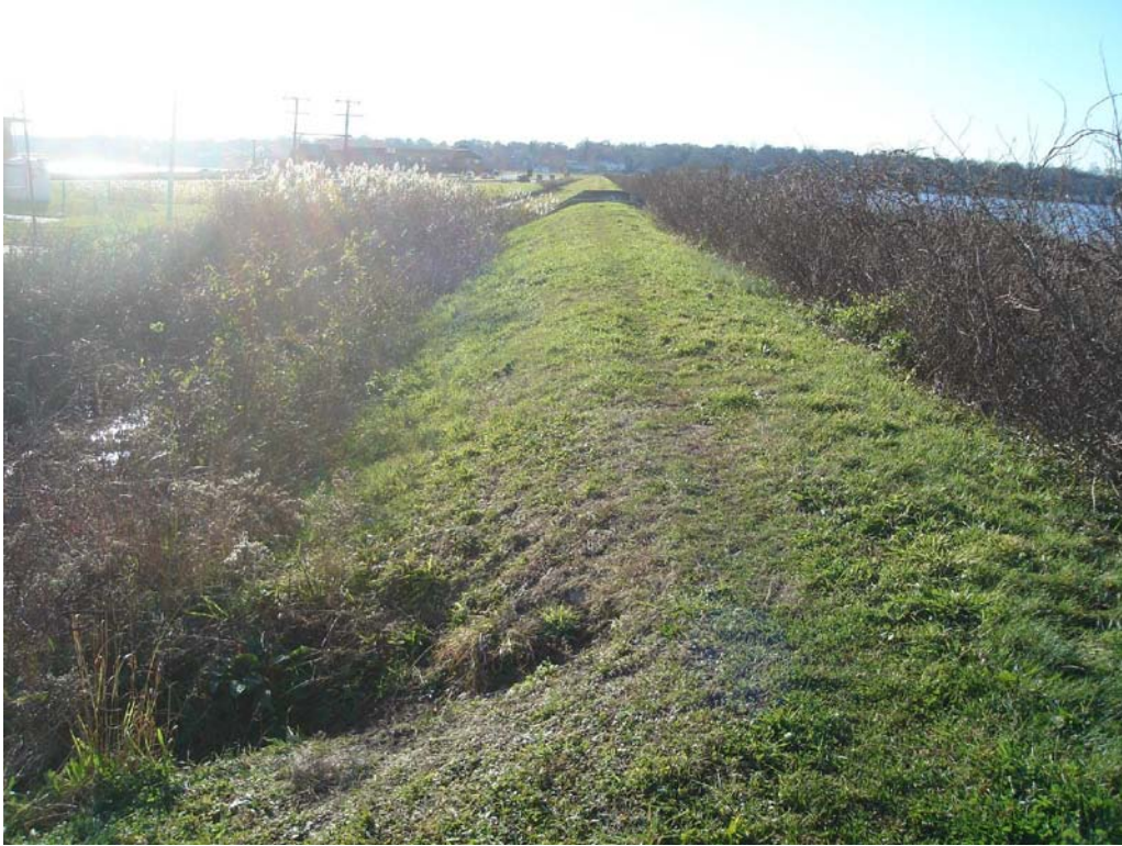
East Embankment - Footpath/erosion rill on downstream slope
