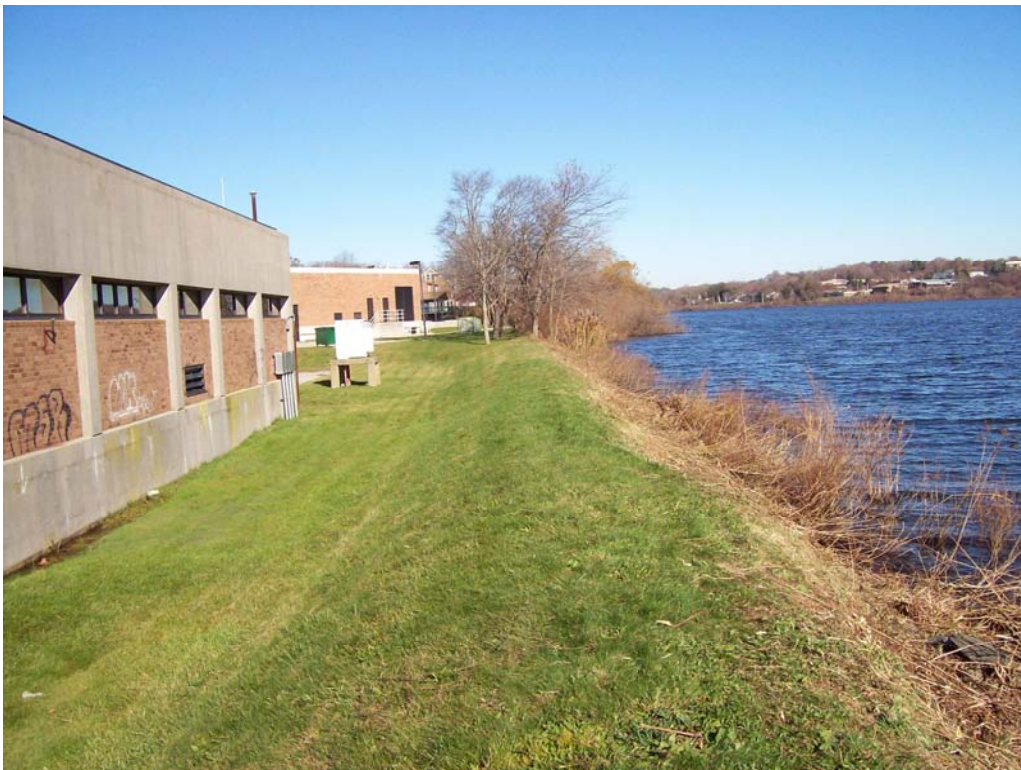
North Pond Embankment – Trees at north end of embankment
