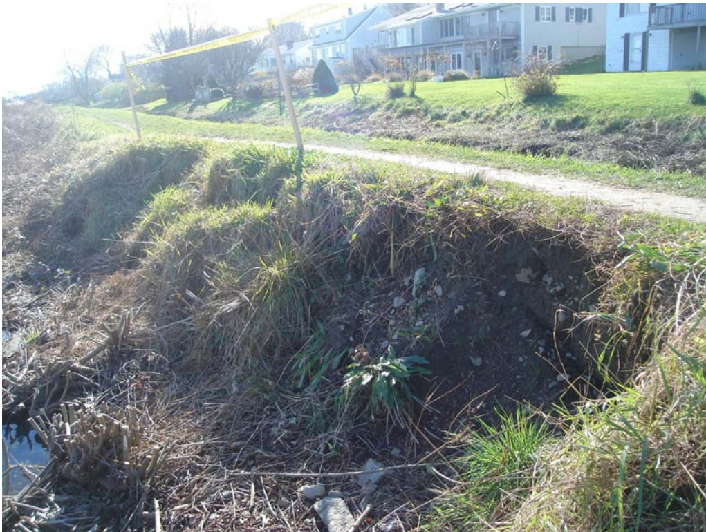
West Embankment – Severe scarps on upstream slope resulting in narrow crest width
