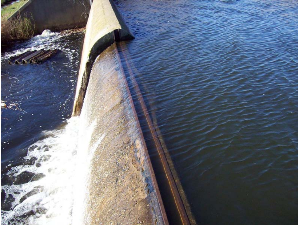
South Pond Spillway - Concrete spalling along spillway weir board rail
