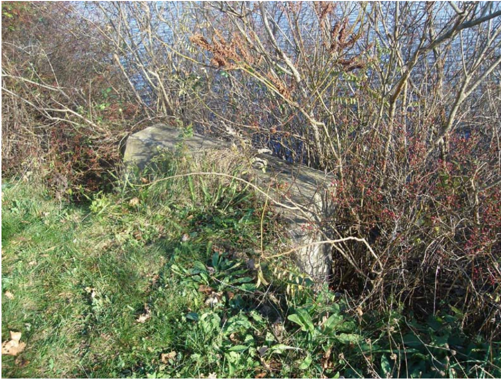
North Pond Embankment – Woody vegetation and scouring along discharge outlet structure
