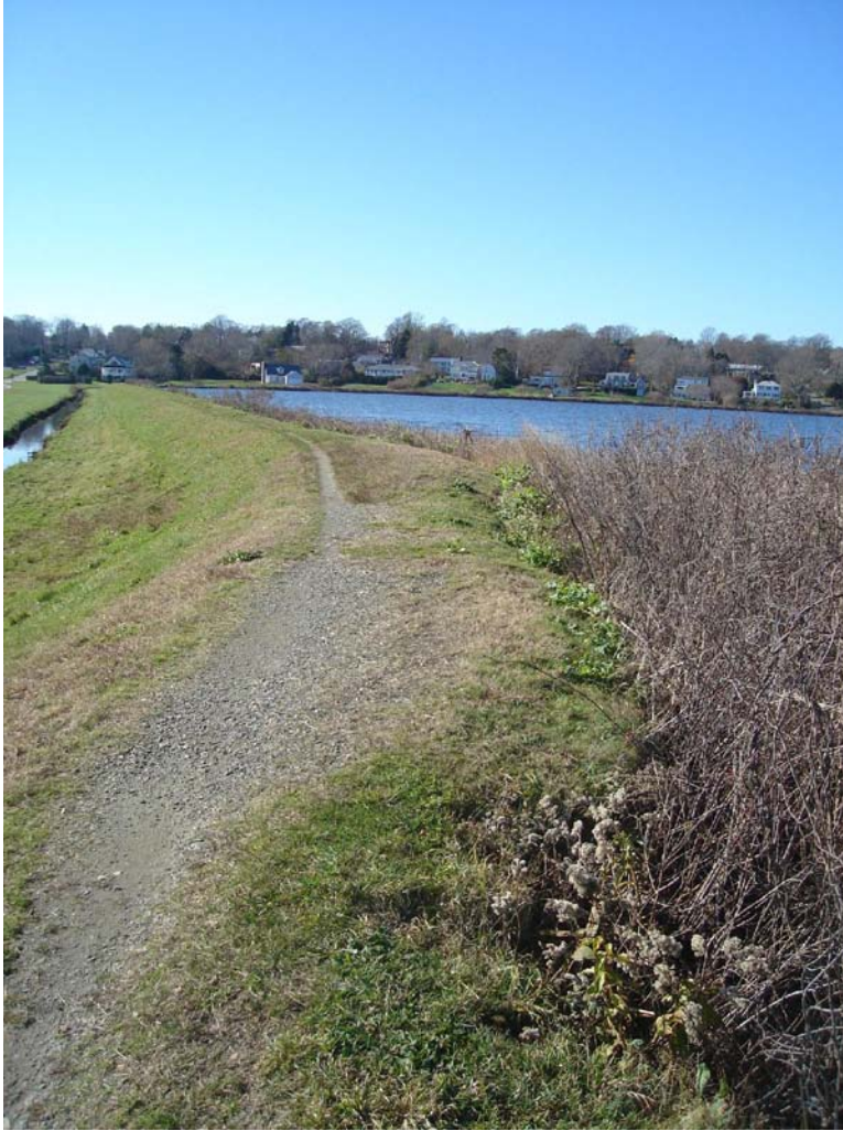
South Embankment – Scarps on upstream slope resulting in narrow crest
