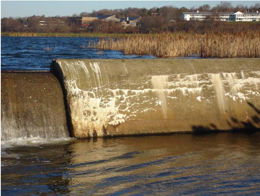
South Pond Spillway - Cracking and efflorescence on face of left downstream spillway
