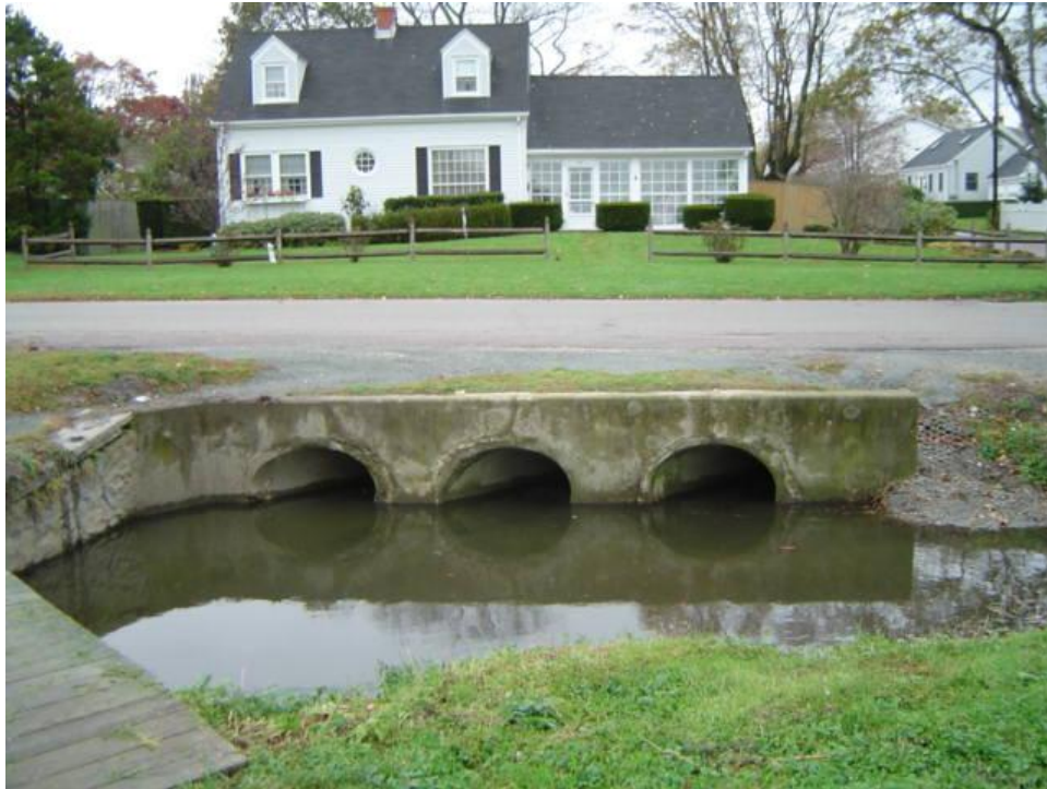
Sta. 62+77: Photo of Moat Just Upstream of Pedestrian Bridge (View of 3-36" Stormwater Outlets Upstream of Bridge)
