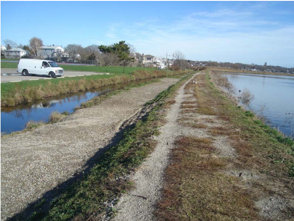
North Embankment – Gravel fill reinforcement on bench along downstream toe of slope
