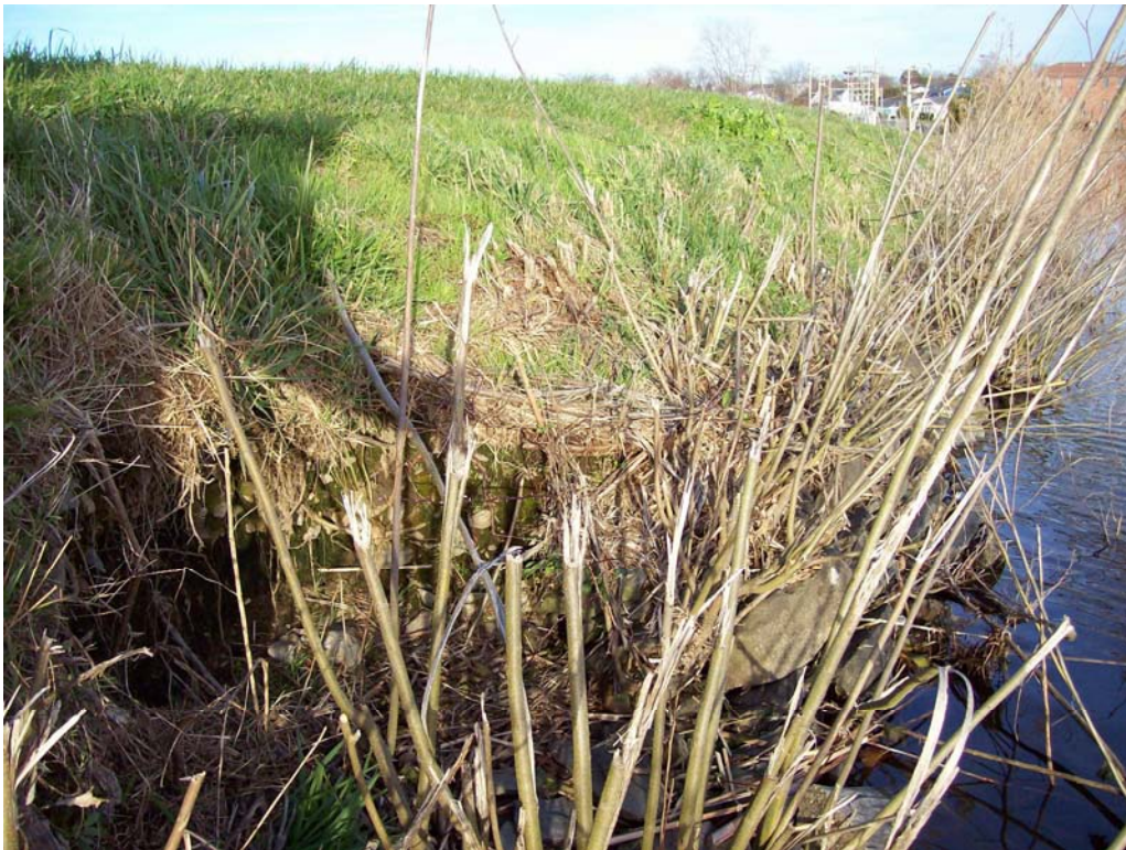
South Pond/North Pond Dividing Embankment – Severe scarp on downstream slope
