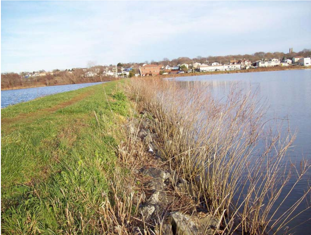
South Pond/North Pond Dividing Embankment –Scarps on downstream slope
