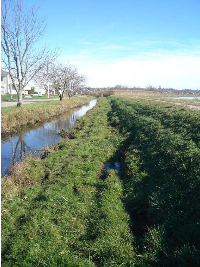
North Embankment – Saturated bench and equipment rilling along moat channel
