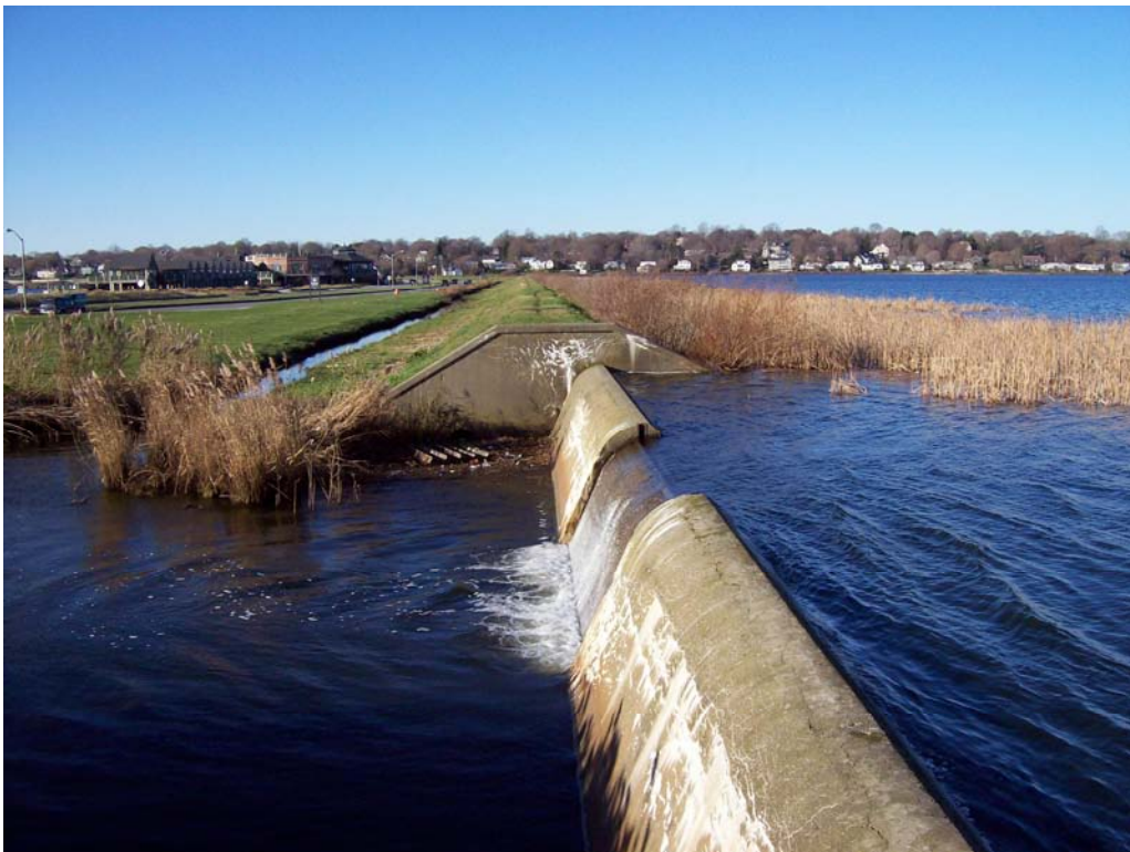
South Pond Spillway - Cracking and efflorescence on face of downstream spillway
