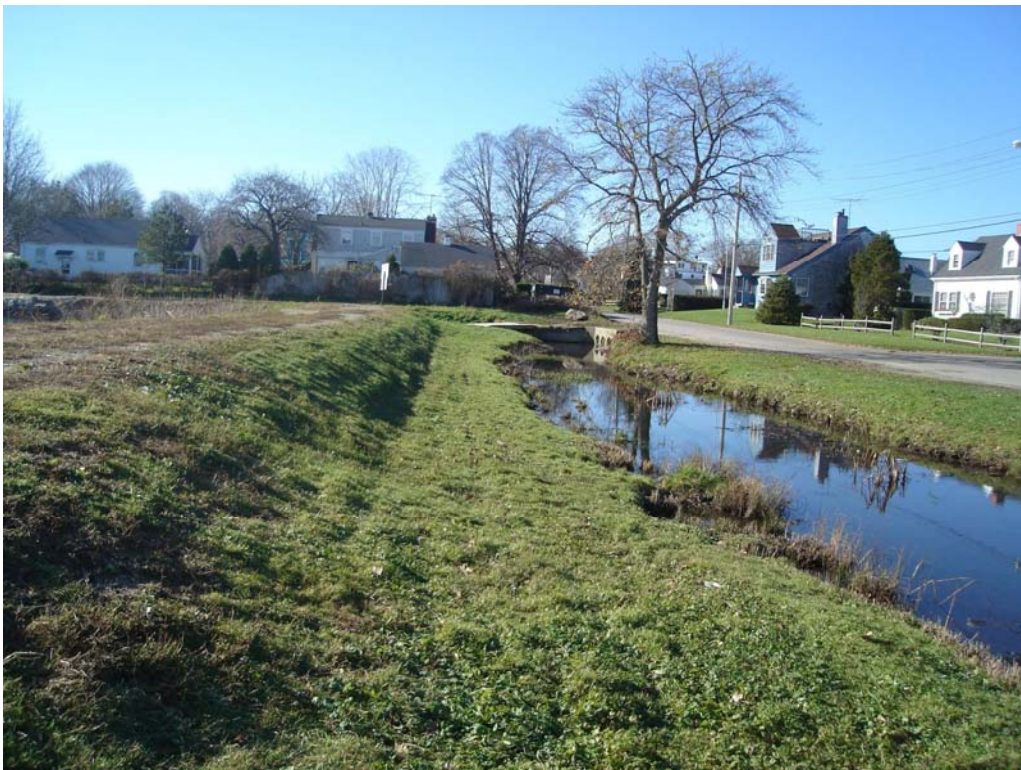
North Embankment – Narrow bench/moat scouring along downstream slope
