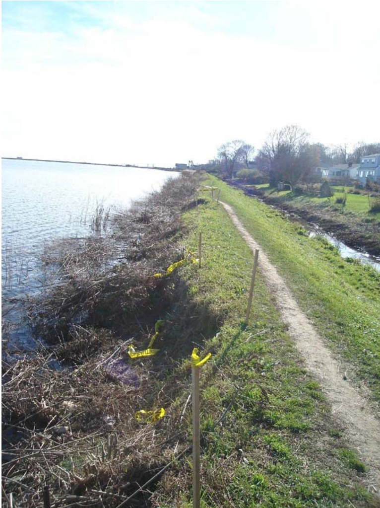
West Embankment – Severe scarps on upstream slope resulting in narrow crest width
