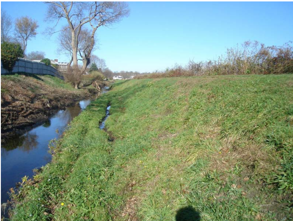
West Embankment – Narrow saturated bench along downstream toe of slope; equipment rutting
