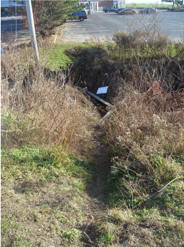
East Embankment – Footpath/erosion rill on downstream slope
