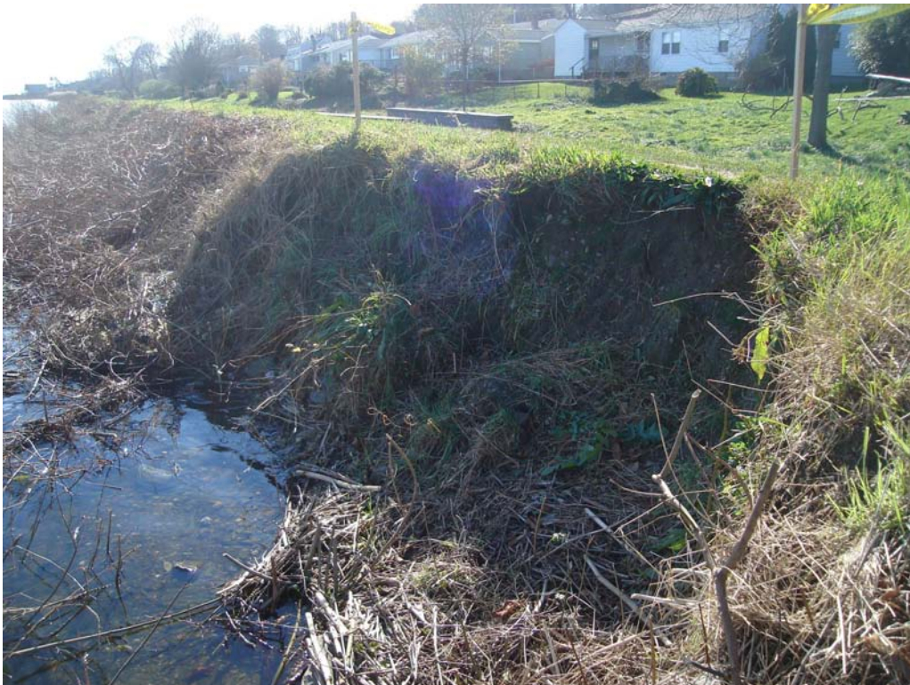
West Embankment – Severe scarp on upstream slope resulting in narrow crest width
