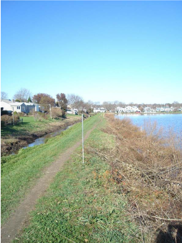
West Embankment – Severe scarps on upstream slope resulting in narrow crest width
