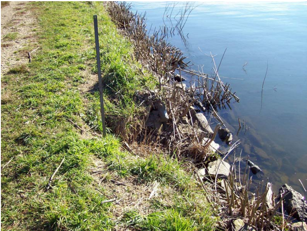
North Embankment – Rilling on upstream slope
