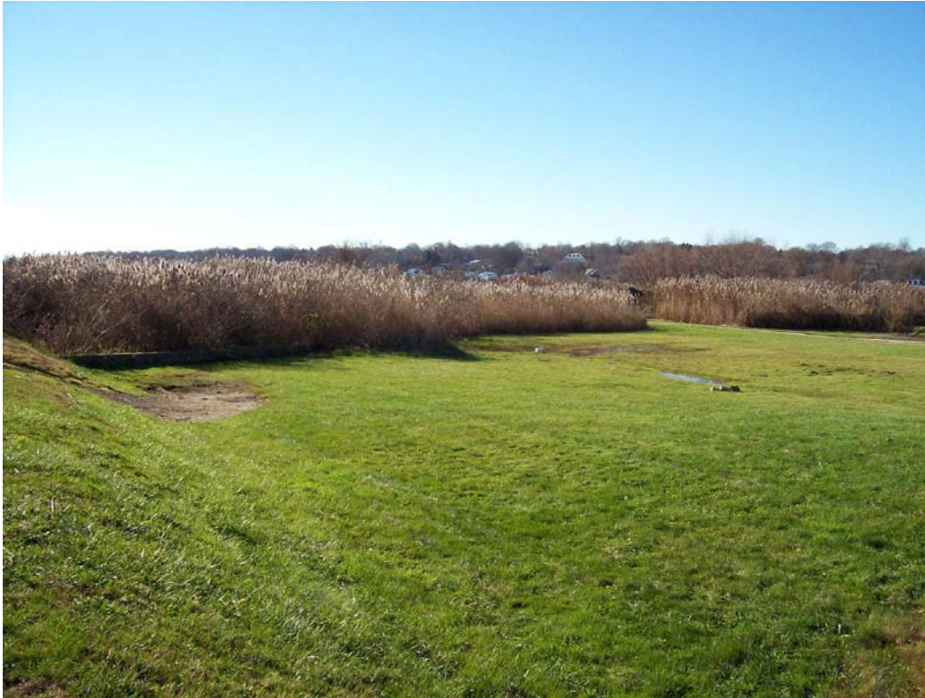
North Pond Embankment — Saturated area with ponding water downstream of North Pond emergency overflow spillway; significant vegetation in downstream channel
