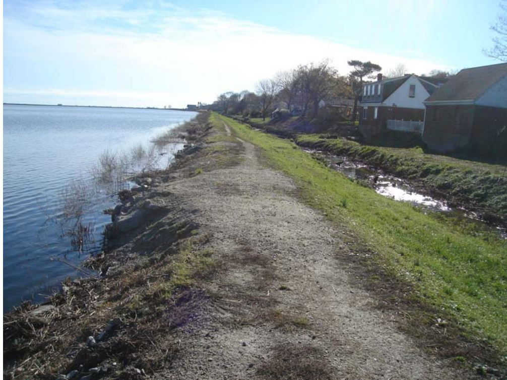
Sta. 62+57: Photo of Moat and Adjacent Pond Embankment (Looking in Downstream Direction)
