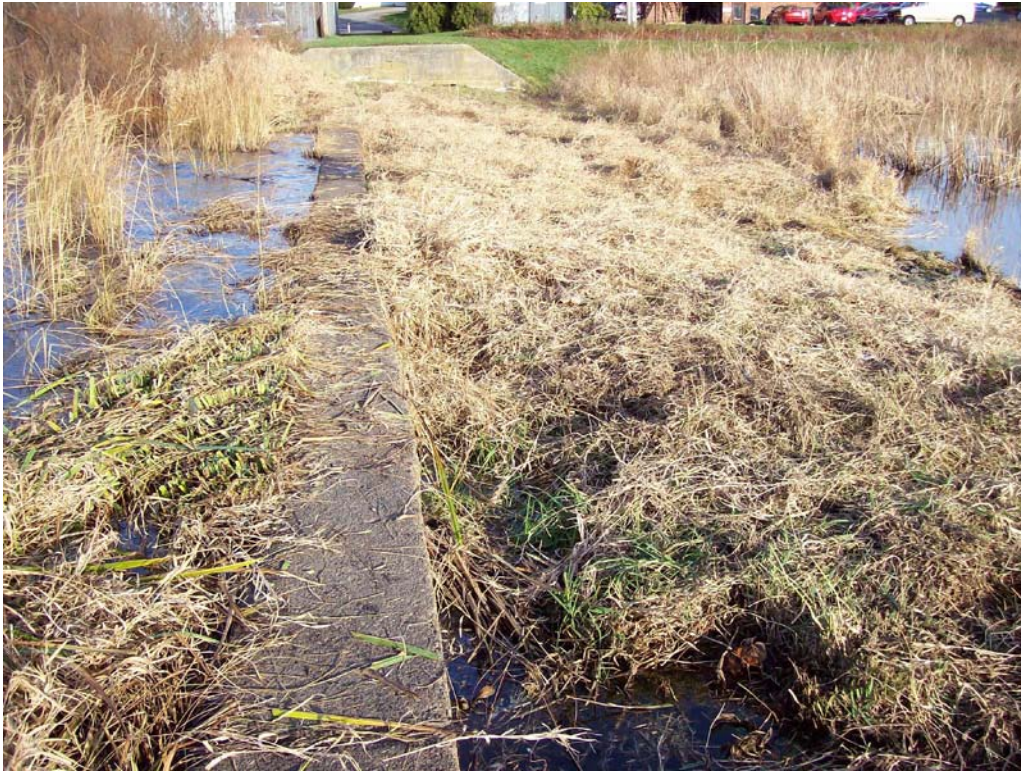
North Pond Primary Spillway - Concrete spillway bar and vegetation; missing scour protection downstream of spillway bar
