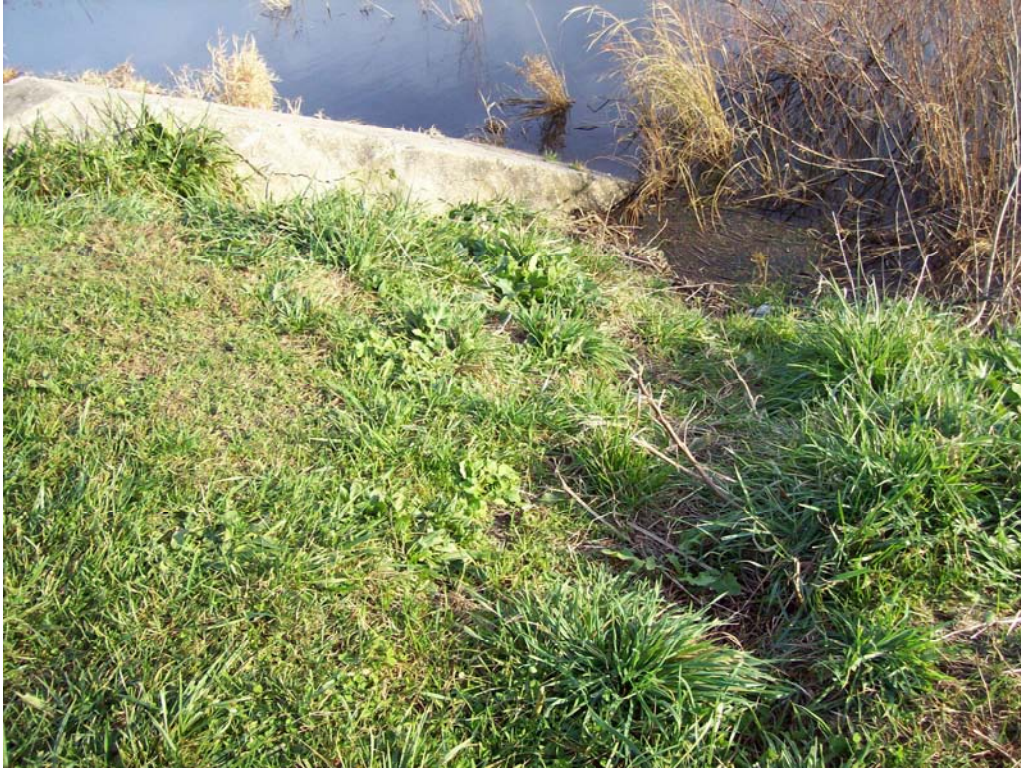
North Pond Primary Spillway - Footpath and runoff channel adjacent to downstream right abutment
