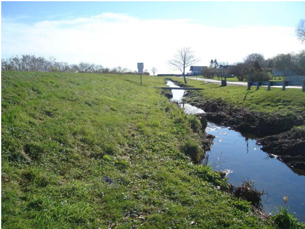
Sta. 41+67: Photo of Moat along Old Beach Road (Looking in Downstream Direction)
