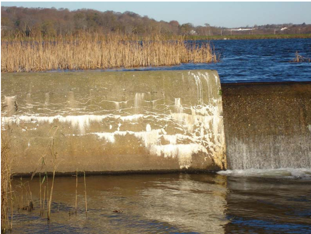
South Pond Spillway - Cracking and efflorescence on face of right downstream spillway
