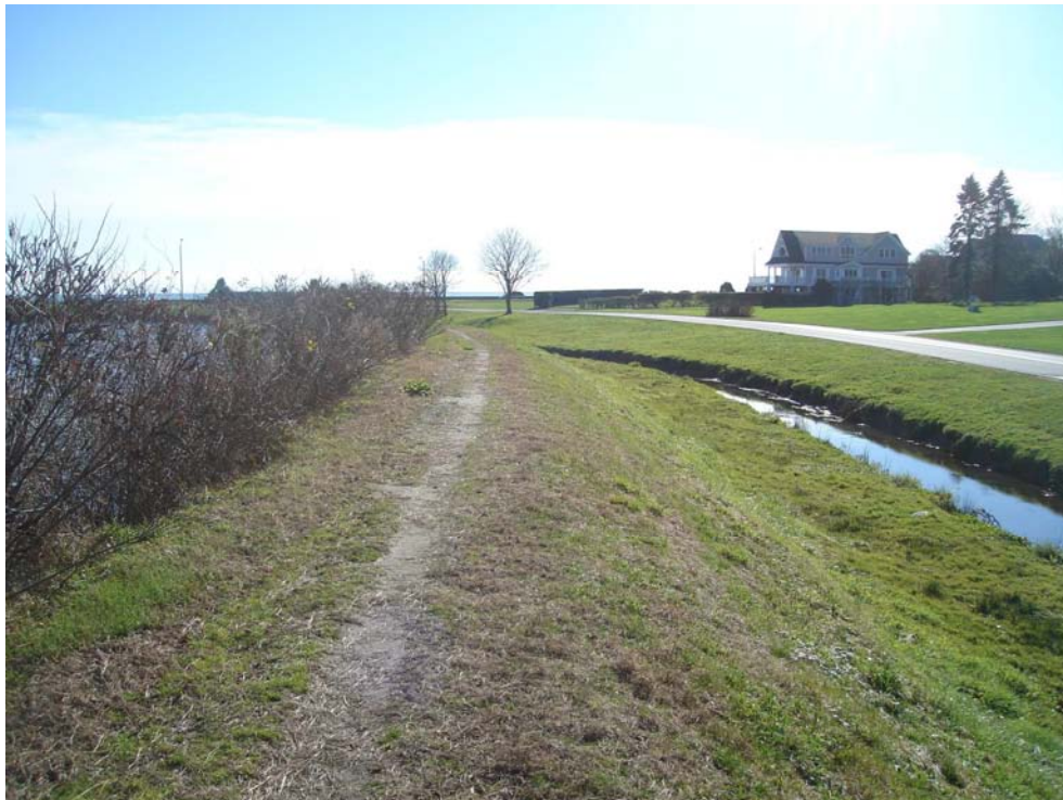
Sta. 36+36: Photo of Moat along Old Beach Road (Looking in Downstream Direction)
