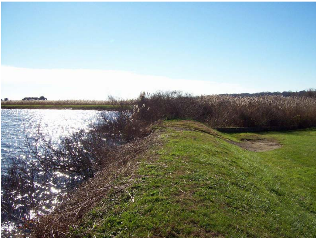
North Pond Embankment – Cleared embankment adjacent to North Pond emergency overflow spillway
