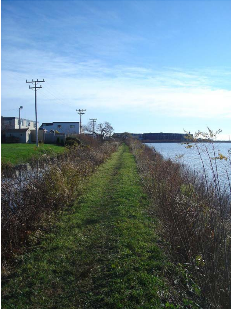
East Embankment –Vegetation on embankment, narrow crest width
