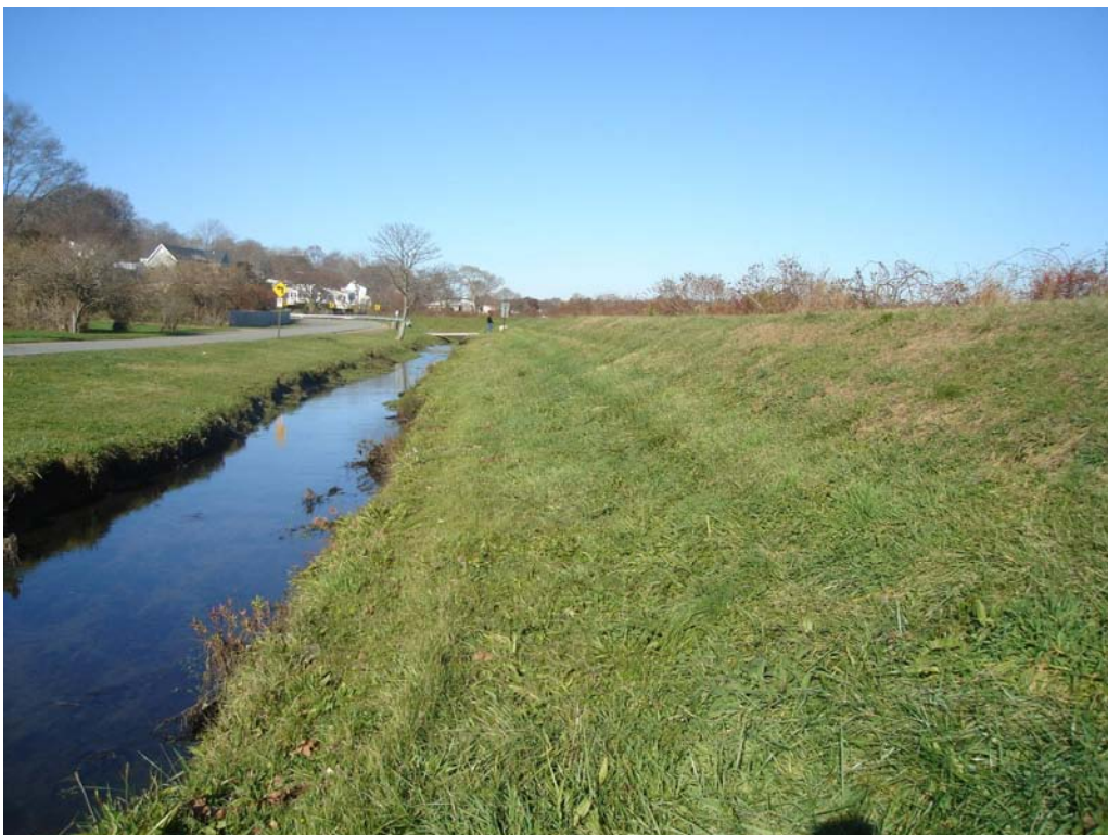
West Embankment - No bench along downstream toe of slope
