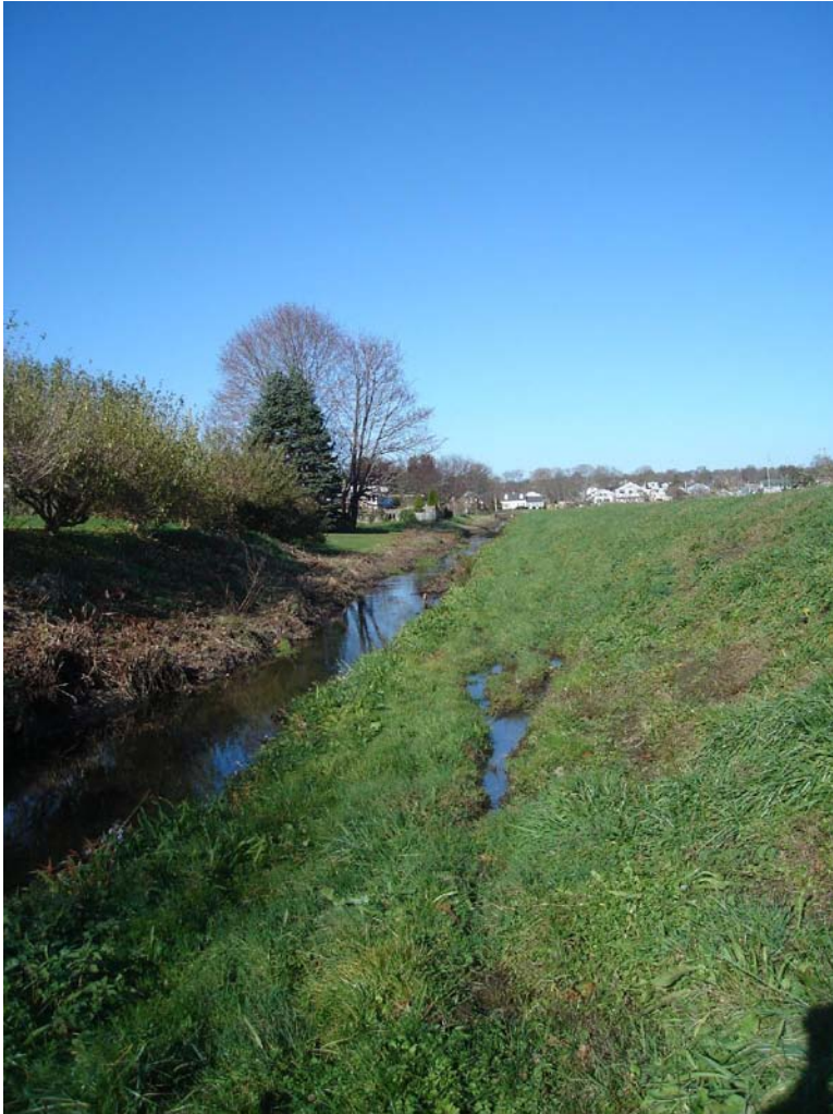
West Embankment – Narrow saturated bench along downstream toe of slope; equipment rutting
