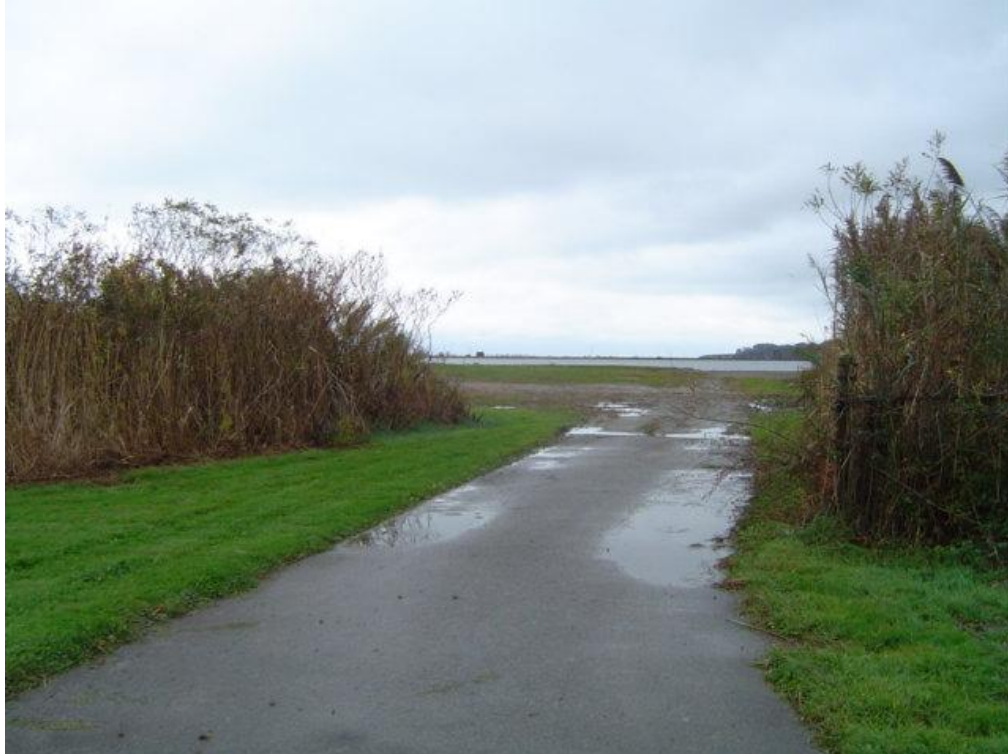
Sta. 77+54 and 77+65: Photo of Access Path at Treatment Facility that Bisects Moat (Downstream of No. Easton Pond Secondary Spillway)
