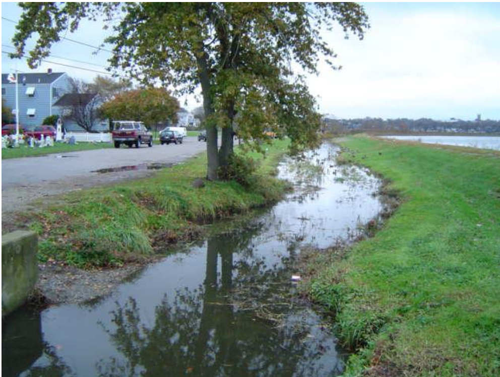
Sta. 62+77: Photo of Moat Upstream of Pedestrian Bridge (Looking in Upstream Direction along Ellery Road)
