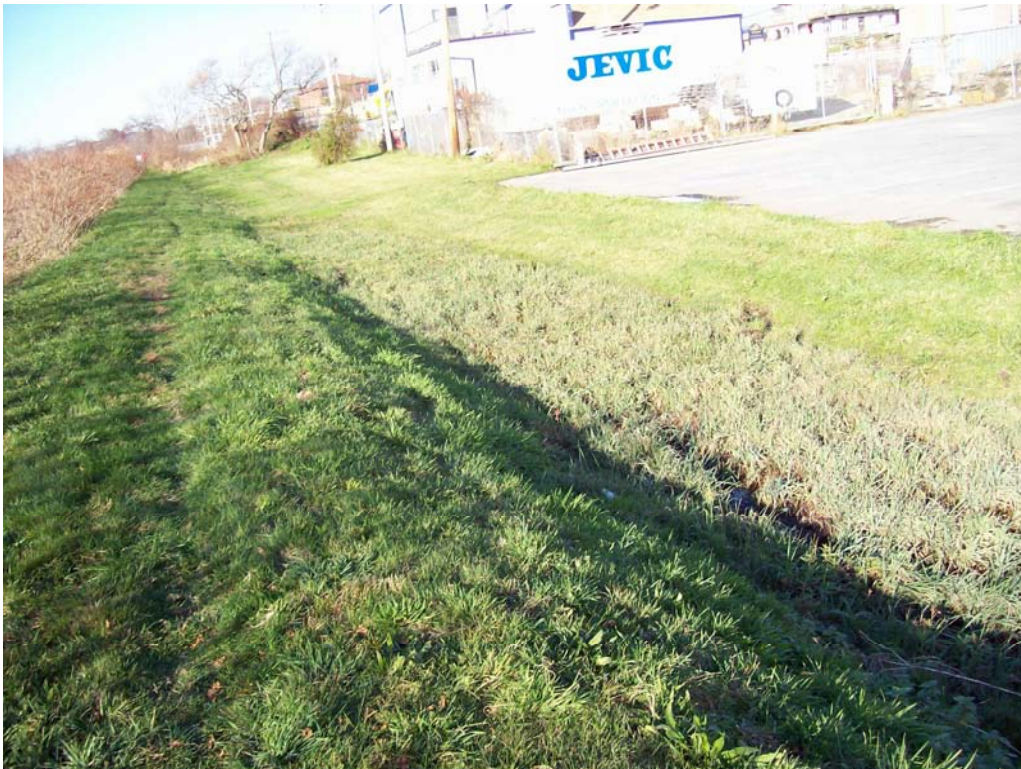
East Embankment – Informal drainage overflow pathway along downstream toe of slope downgradient of submerged channel outlet
