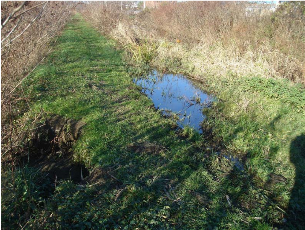
East Embankment – Drainage channel near submerged culvert outlet overflowing embankment crest resulting in erosion and scarp on upstream embankment.
