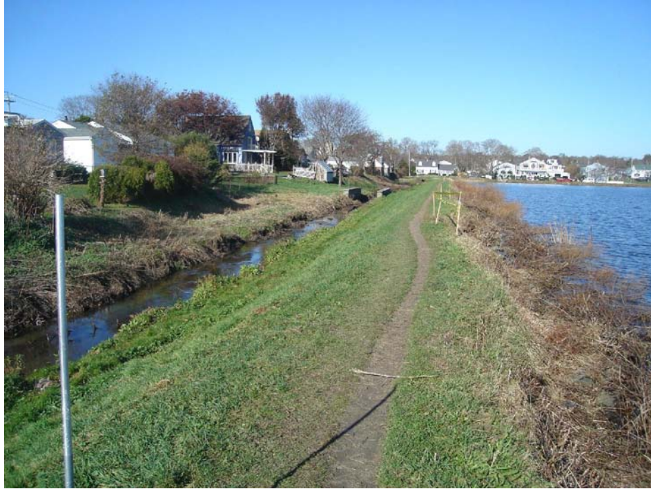
Sta. 50+21: Photo of Moat and Adjacent Pond Embankment (Looking in Upstream Direction)
