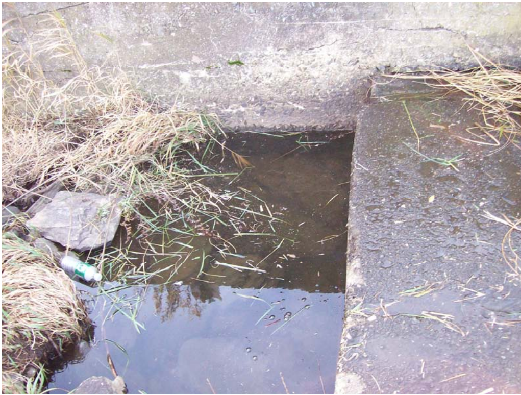
North Pond Primary Spillway - Missing scour protection downstream of spillway bar at junction with right abutment
