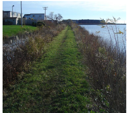
Photograph 12: Narrow Crest Width on East Embankment
