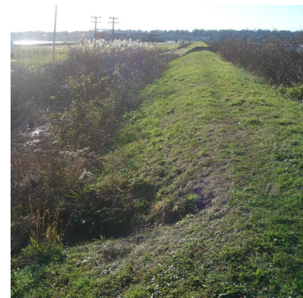
Photograph 8: Worn Footpath Causing Erosion on East Embankment
