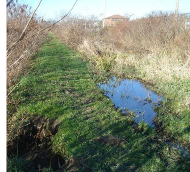
Photograph 5: Rilling/Scarp on East Embankment (Standing Water Obscured in Background)
