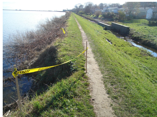
Photograph 11: Upstream Slope Failure and Worn Footpath on West Embankment
