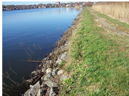
Photograph 13: Upstream Slope Protection and Worn Footpath on North Embankment
