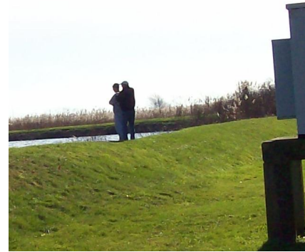
Photograph 7: North Pond Embankment Settlement Area
