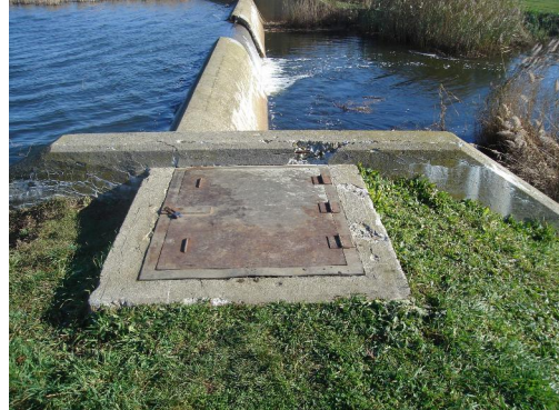
Photograph 4: Deteriorating Concrete at South Pond Spillway
