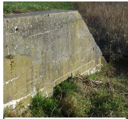
Photograph 3: Void at Bottom of Left Abutment
