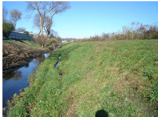
Photograph 9: Moat Encroachment and Bench Rutting along West Embankment
