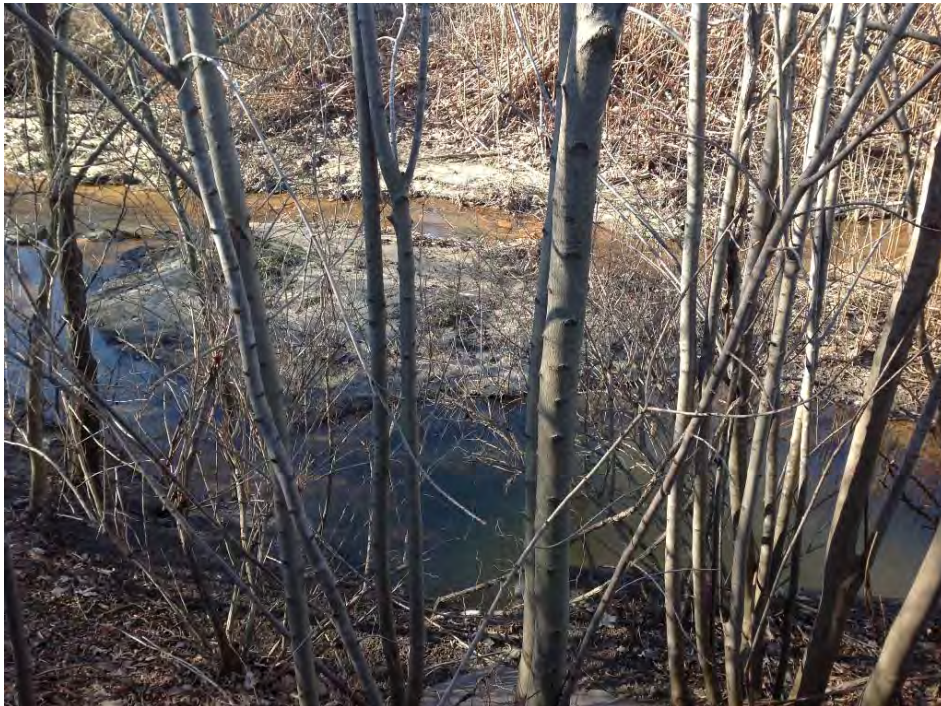
Photo 2: Drainage channel west of City Yard at 42" outfall from DMH-037-2A (looking west), vegetation, debris, and sediment visible (01/09/2014)
