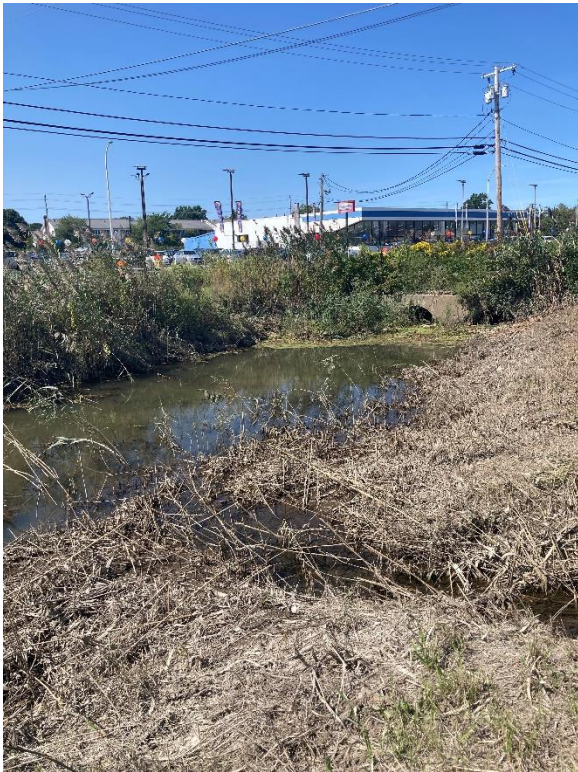
Photo 7: Culvert DP-025-7 (looking northwest) taken looking at the crossing under JT Connell Hwy (05/26/2022)
