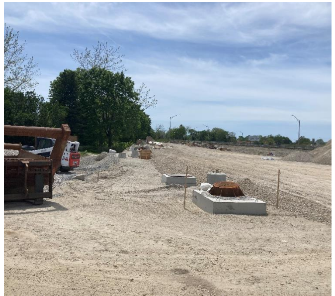
Photo 8: Pell Bridge Project construction progress (looking southwest) taken at the end of Halsey St (05/26/2022)
