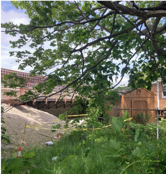
Photo 9: Pell Bridge Project retaining wall construction progress (looking north) taken at Prescott Hall Rd and Garfield St (05/26/2022)
