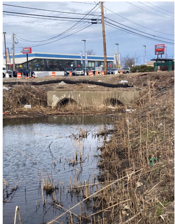
Photo 4: Culvert DP-025-7 (looking northwest) taken looking at the crossing under JT Connell Hwy (02/24/2022)
