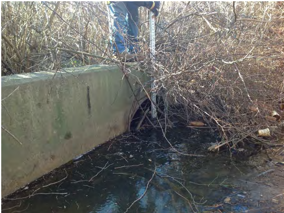
Photo 4: Downstream headwall (looking west) of 42" storm drain from State 138/238, discharges into southern end of drainage channel located immediately west of City Yard. Vegetation and debris visible (01/09/2014).
