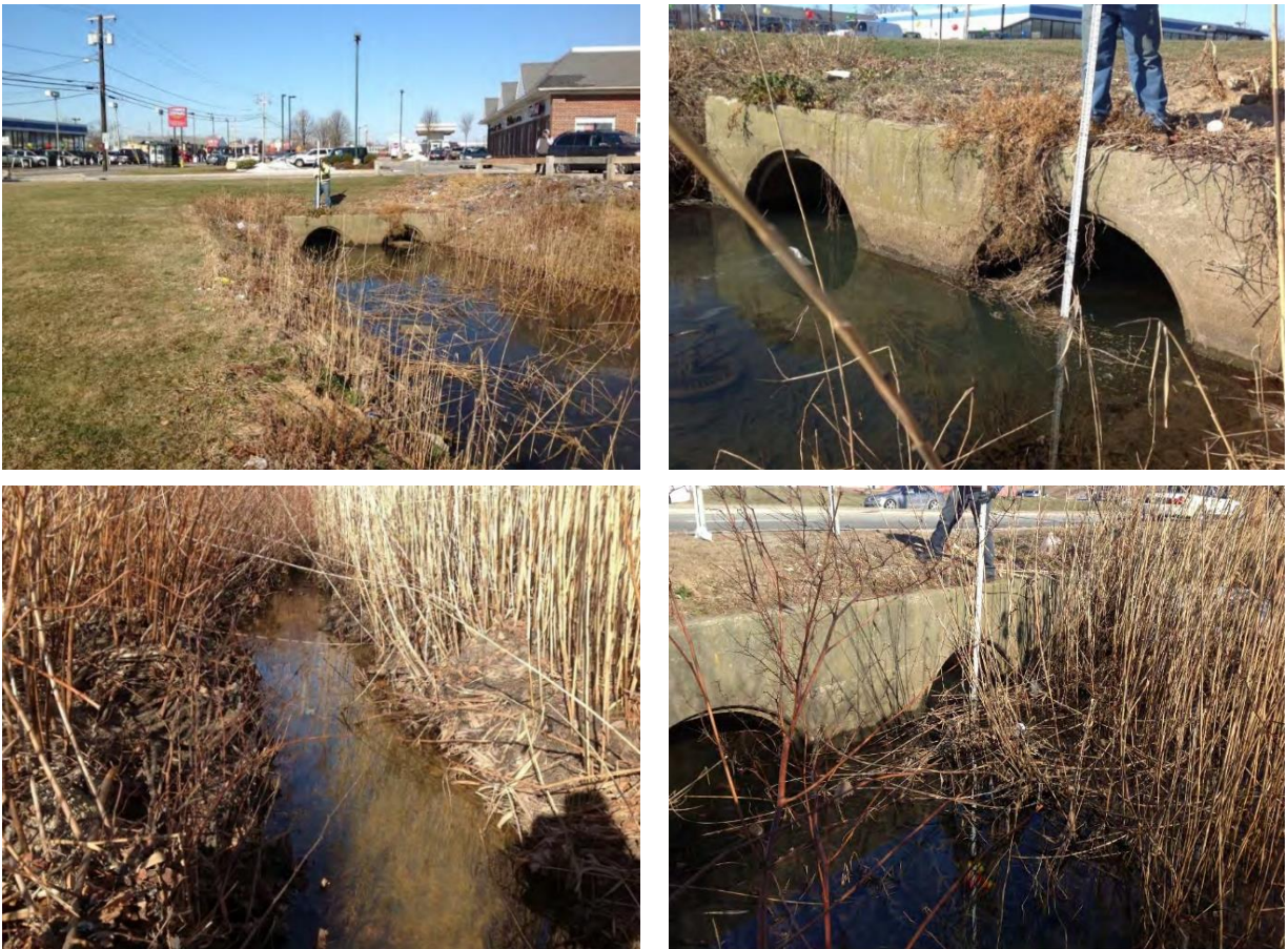
Figure 2-3. RIDOT Open Channels and Culverts Along JT Connell Highway ( photos taken in January 2014 )
