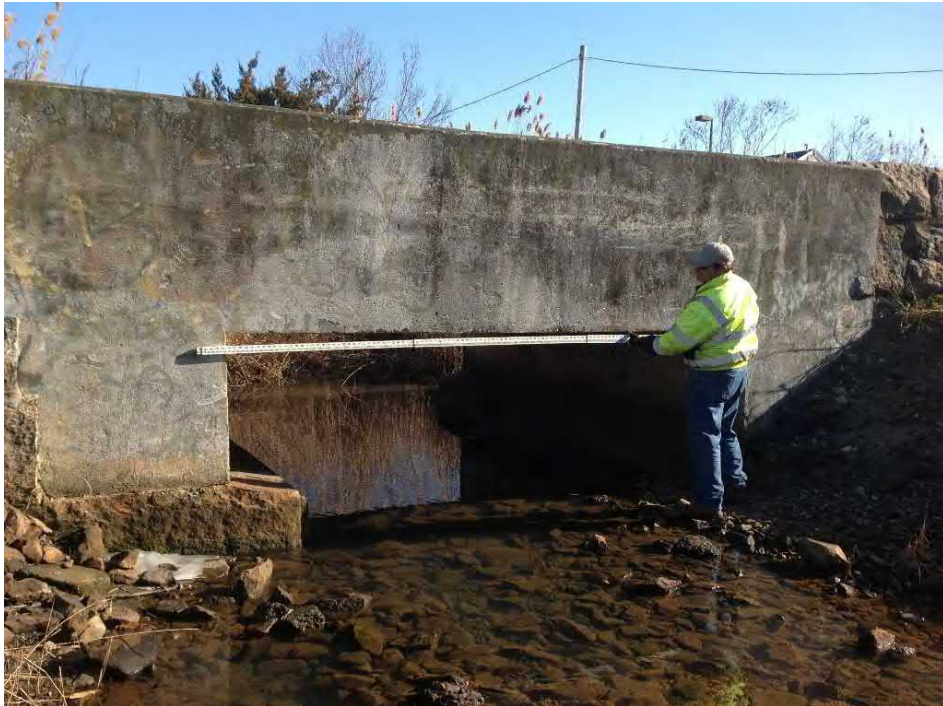
Photo 17: Downstream side of 12' railroad box culvert (looking east), drainage channel continues to Newport Harbor. (01/09/2014)
