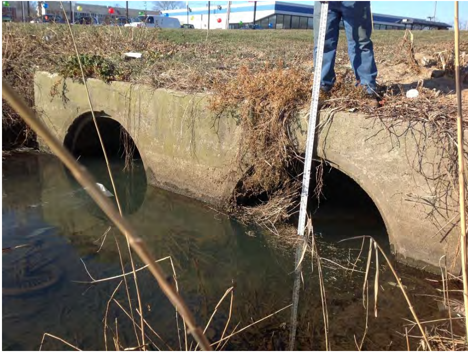
Photo 14: Upstream headwall at north end of drainage channel at northeast corner of Kalbfus/JT Connell rotary, twin 60" pipe culverts, debris and vegetation visible. Pipe invert elevations appear to be higher than the pipe invert elevations at channel inlet (Photo 12). (01/09/2014)
