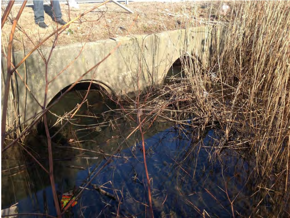
Photo 12: Downstream headwall for twin 60" pipe culvert under rotary (looking south) at intersection of Admiral Kalbfus and JT Connell Highway, vegetation visible. (01/09/2014).
