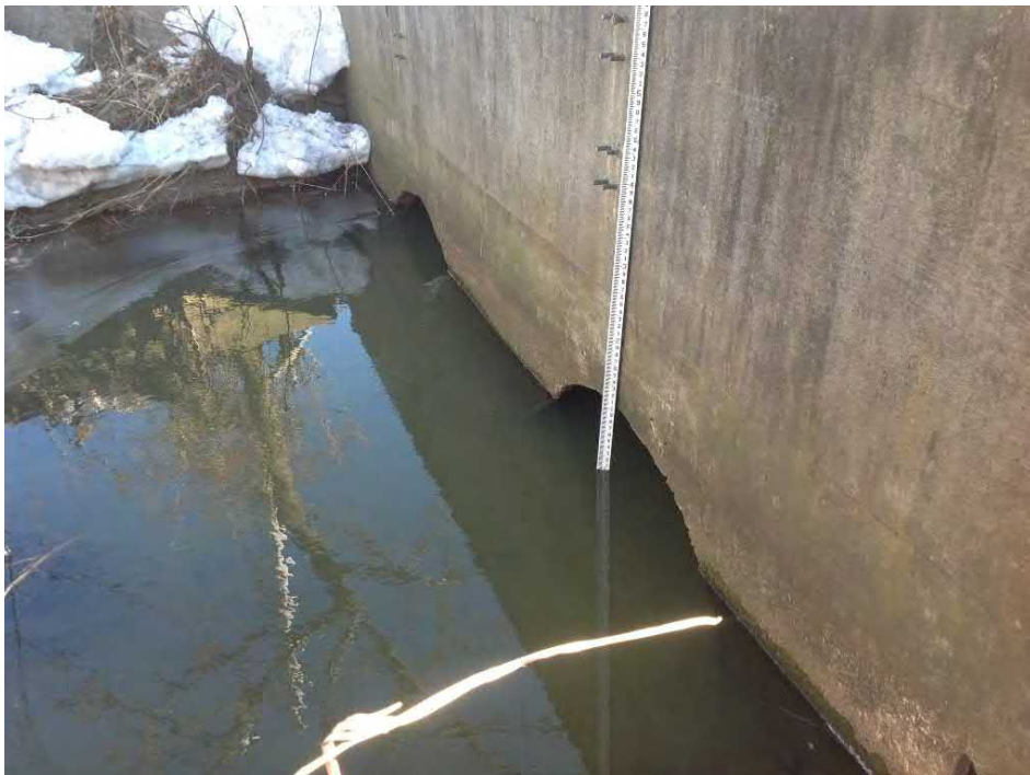
Photo 15: Downstream headwall of twin 60" pipe culvert west of JT Connell Highway (rear of car dealership at 116 JT Connell Highway). (01/09/2014)
