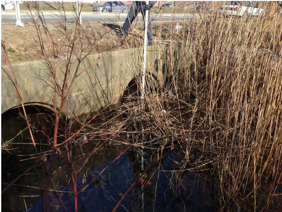
Photo 11: Upstream headwall for twin 60" pipe culvert under rotary (looking north) at intersection of Admiral Kalbfus and JT Connell Highway, vegetation visible. (01/09/2014).
