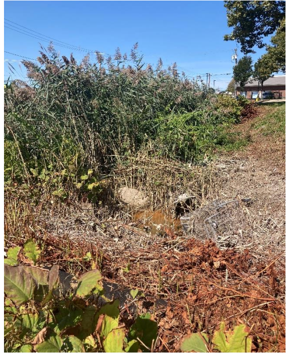
Photo 6: Drainage Channel DP-025-8 (looking northeast) taken after the crossing under Admiral Kalbfus Rd (05/26/2022)
