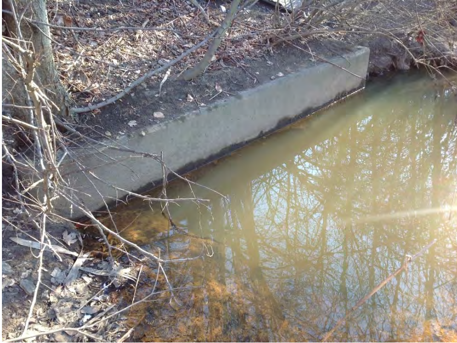
Photo 3: Downstream headwall (looking east) of 42" storm drain from Prescott Hall, pipe crown submerged (01/09/2014).
