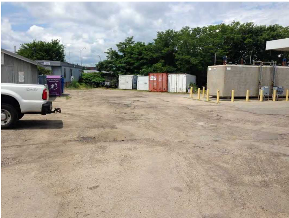
Photo 23: City Yard (looking west from southeast of fuel island), proposed Halsey Street storm culvert would discharge into drainage channel behind storage containers. (06/20/2014)
