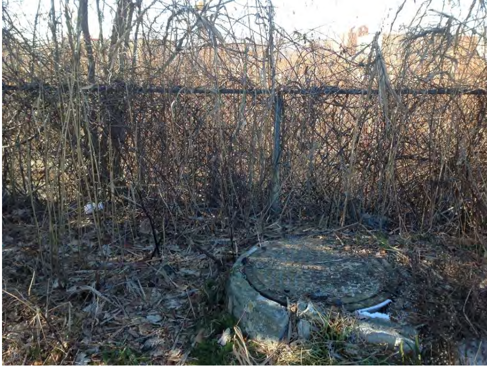
Photo 1: Drainage Manhole DMH-037-2A (looking west) located on western side of City Yard, upstream is 42" storm drain from Prescott Hall, downstream is 42" (assumed) outlet into drainage channel (01/09/2014)
