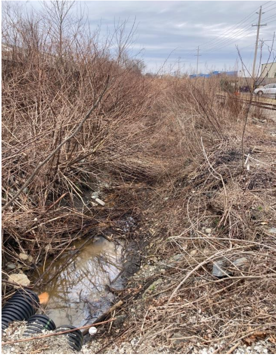
Photo 1: Drainage Channel DP-19-1 (looking north) taken on the northern side of the crossing under Admiral Kalbfus Rd (02/24/2022)
