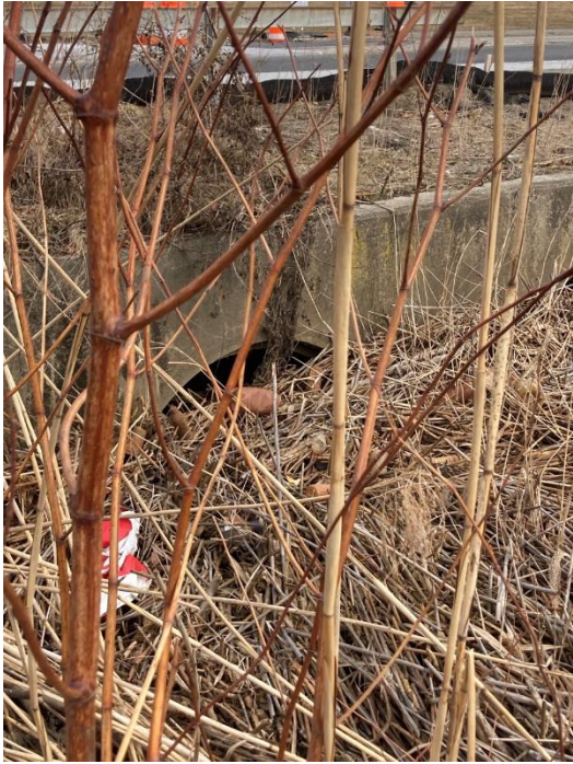
Photo 5: Culvert DP-025-13 (looking northwest) taken looking at the crossing under Admiral Kalbfus Rd (02/24/2022)
