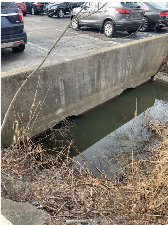
Photo 3: Culvert DP-025-7 (looking southeast) taken looking at the crossing under car dealership parking lot (02/24/2022)
