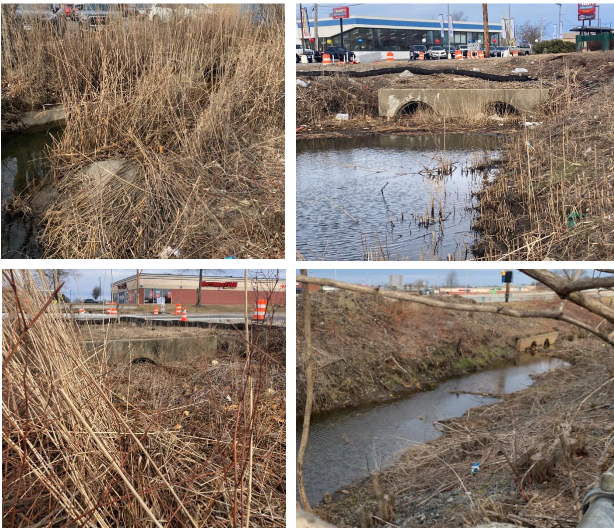
Figure 3-1. State Open Channels and Culverts Along JT Connell Highway (photos taken in February 2022)
