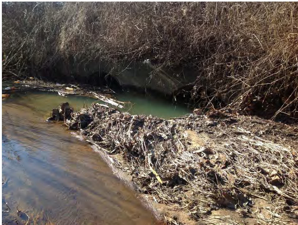
Photo 6: Drainage channel west of City Yard, upstream headwall for twin 60" pipe culverts, vegetation, debris, and sediment visible (01/09/2014)
