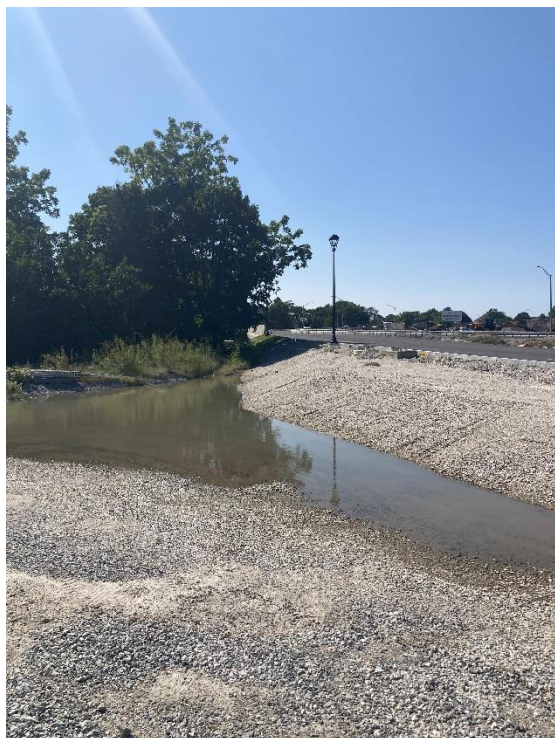
Photo 11: Pell Bridge Project Construction Progress (looking southwest) taken at the end of Halsey St (09/18/2022)
