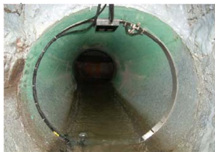
Meter CH-02 on Wellington Avenue Post-Wellington Interceptor Replacement
