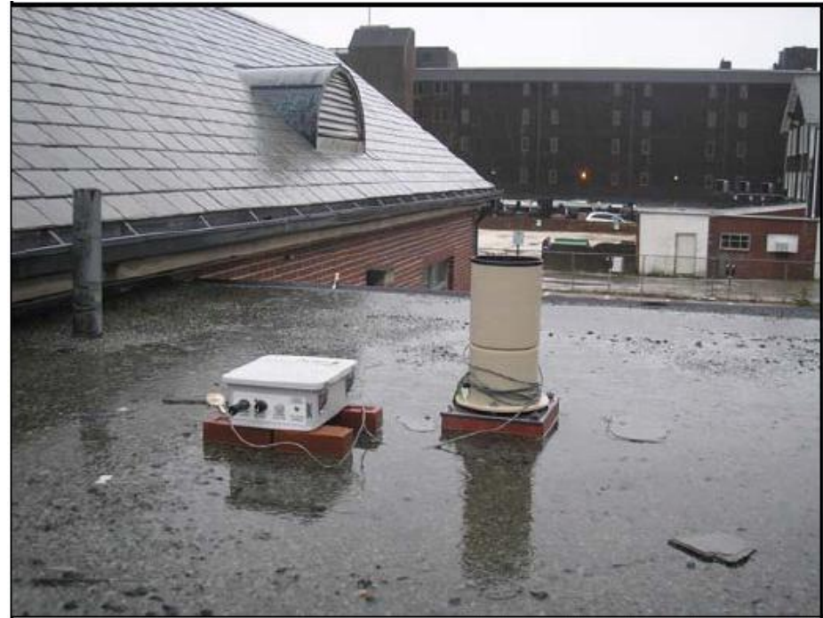
Rain gage at Long Wharf Pump Station
