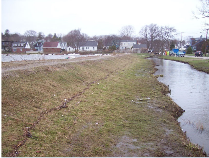
Figure 7 – Moat Channel along South Easton Pond North Embankment Spillway Structure (Post-Storm, April 2007)
