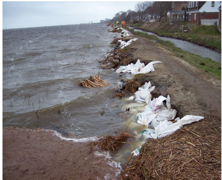
Figure 3 – Emergency Repairs to Damaged South Easton Pond West Embankment in April 2007 North and South Easton Ponds
