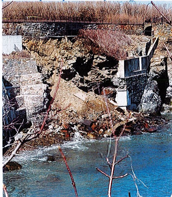
Collapsed Section of Cliff Walk
