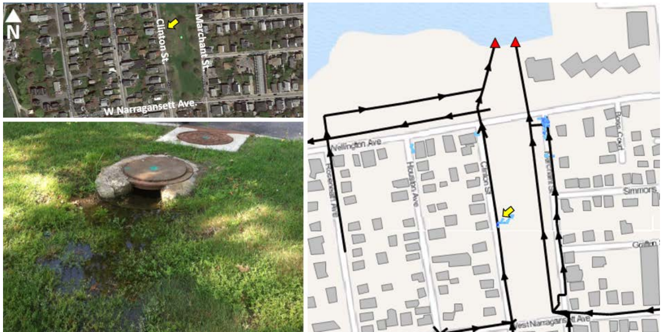
Figure 3-6. Wellington Avenue Dry Weather Flooding Validation Event This event was a high tide on Sept. 1, 2015 of 5.0 feet (MLLW) seen in the field, no rain
