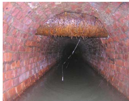
PHOTOGRAPH 3.2: Upstream view of a cast iron pipe running through the crown of the interceptor at Dean Street.
