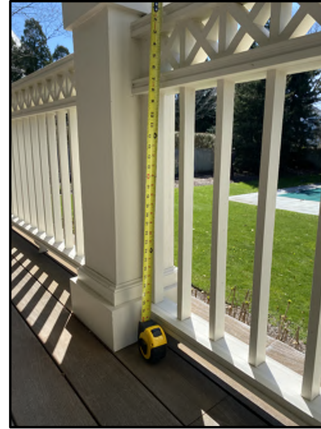
SOUTH ELEVATION GROUND FLOOR REAR DECK EXISTING DECK RAILING BOTTOM RAIL TO BE MATCHED
