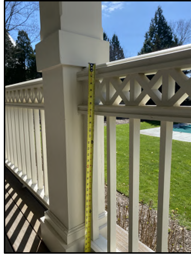
SOUTH ELEVATION GROUND FLOOR REAR DECK EXISTING DECK RAILING TOP RAIL TO BE MATCHED
