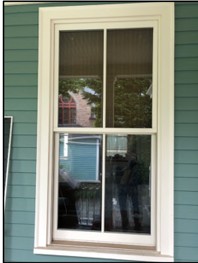
EAST ELEVATION FIRST FLOOR FAMILY ROOM EXISTING DOUBLE HUNG WINDOW TO BE REPLACED TO MATCH EXISTING
