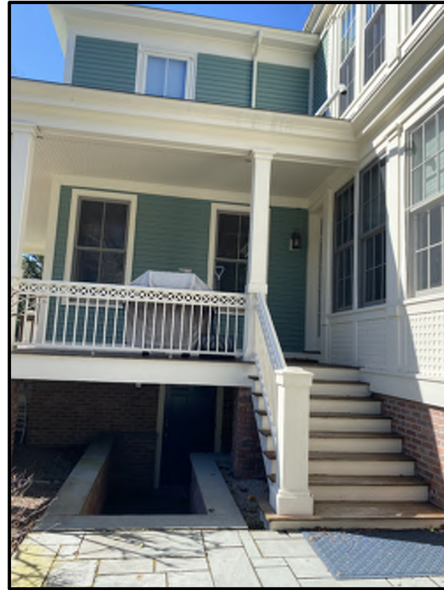
EAST ELEVATION FIRST FLOOR FAMILY ROOM LOCATION OF NEW FRENCH DOORS AND SCREEN DOORS
