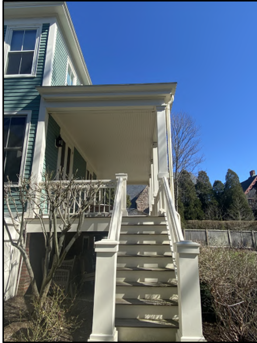
WEST ELEVATION GRADE LEVEL REMOVE NARROW STAIR TO REAR DECK RECONFIGURE MORE GENEROUS STAIR AT SOUTH ELEVATION. MATCH ALL EXISTING MATERIALS AND PROFILES
