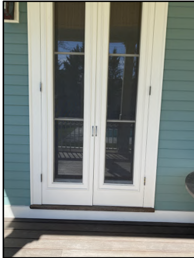
SOUTH ELEVATION FIRST FLOOR FAMILY ROOM EXISTING FRENCH SCREEN DOOR TO BE MATCHED
