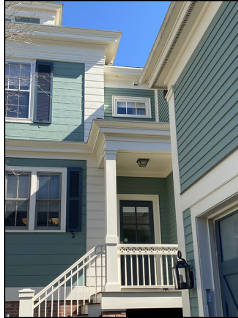
WEST ELEVATION SECOND FLOOR REPLACE 3-LITE AWNING WINDOW WITH 6 OVER 6 DOUBLE HUNG WINDOW TO MATCH EXISTING
