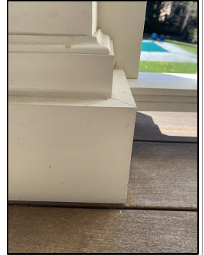
SOUTH ELEVATION GROUND FLOOR REAR DECK EXISTING DECK RAILING POST BASE TO BE MATCHED
