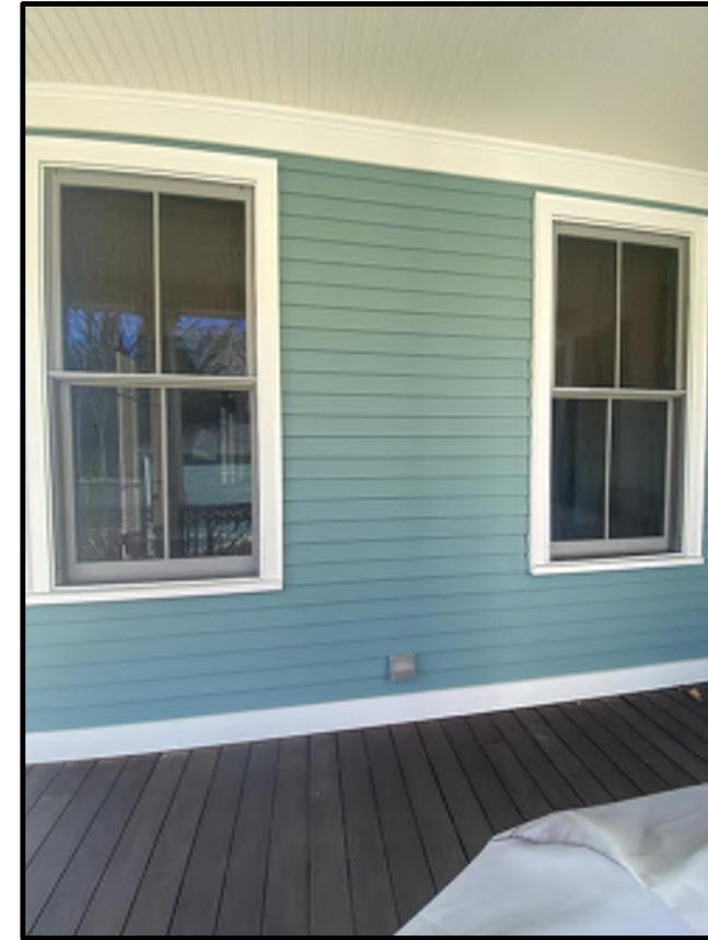
EAST ELEVATION FIRST FLOOR FAMILY ROOM LOCATION OF NEW FRENCH DOORS AND SCREEN DOORS
