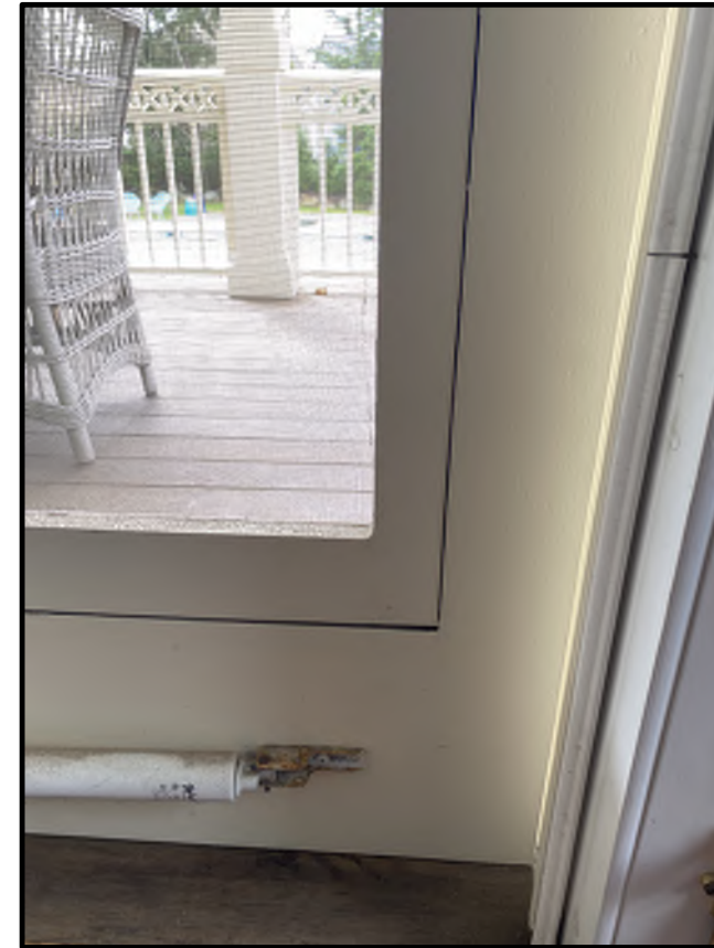
SOUTH ELEVATION FIRST FLOOR FAMILY ROOM EXISTING FRENCH SCREEN DOOR BOTTOM RAIL (INTERIOR) TO BE MATCHED
