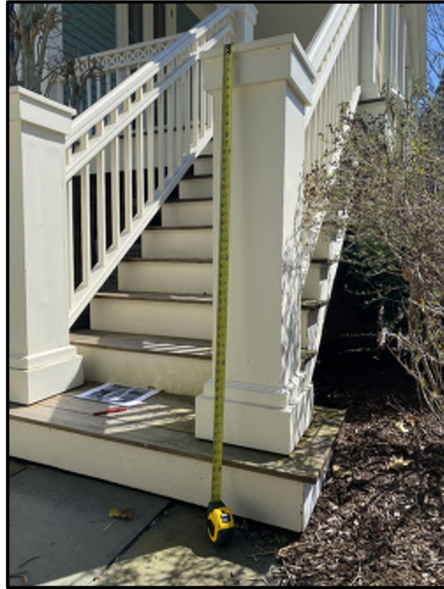
WEST ELEVATION GROUND FLOOR REAR DECK EXISTING NEWEL POST TO BE MATCHED
