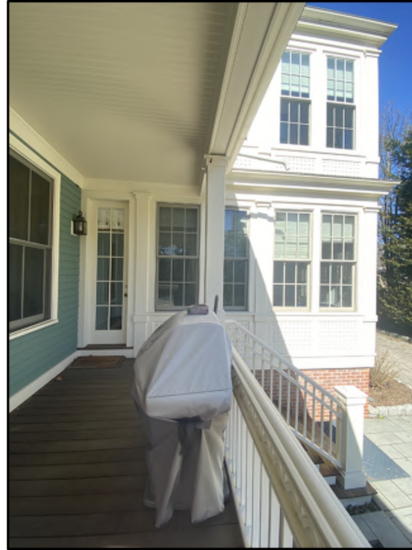
SOUTH ELEVATION FIRST FLOOR REPLACE NARROW 10 LITE FRENCH DOOR WITH 6 OVER 6 DOUBLE HUNG WINDOW TO MATCH ADJACENT
