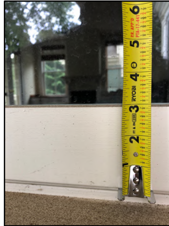
EAST ELEVATION FIRST FLOOR FAMILY ROOM EXISTING DOUBLE HUNG WINDOW BOTTOM RAIL
