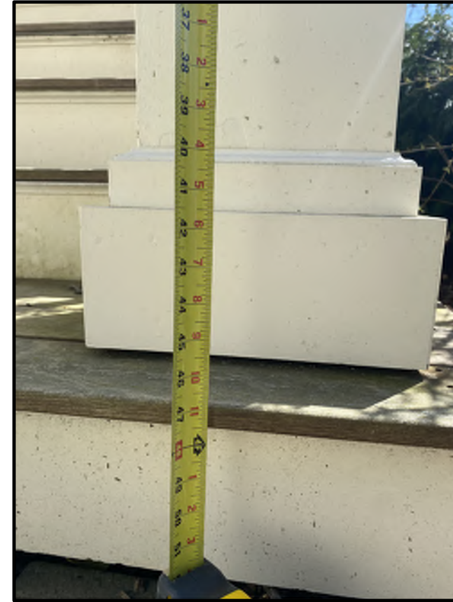
WEST ELEVATION GROUND FLOOR REAR DECK EXISTING NEWEL POST BASE TO BE MATCHED
