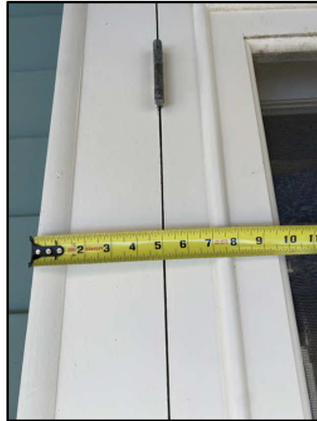
SOUTH ELEVATION FIRST FLOOR FAMILY ROOM EXISTING FRENCH SCREEN DOOR TO BE MATCHED
