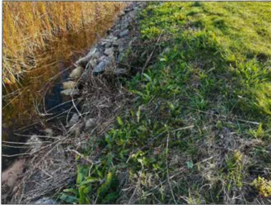
Photo No. 13.: Bowl/depression in the upstream slope near STA 10+40. Typical of the depressions throughout the upstream slope.
