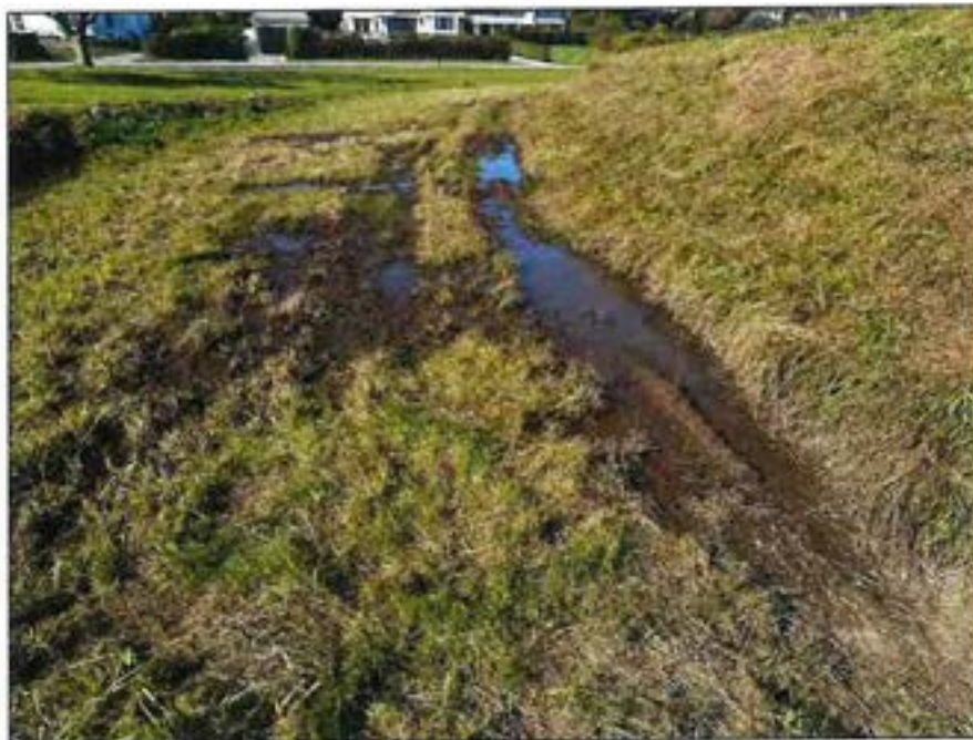
Photo No. 25.: Saturated toe and downstream area near STA 28+00 looking right.
