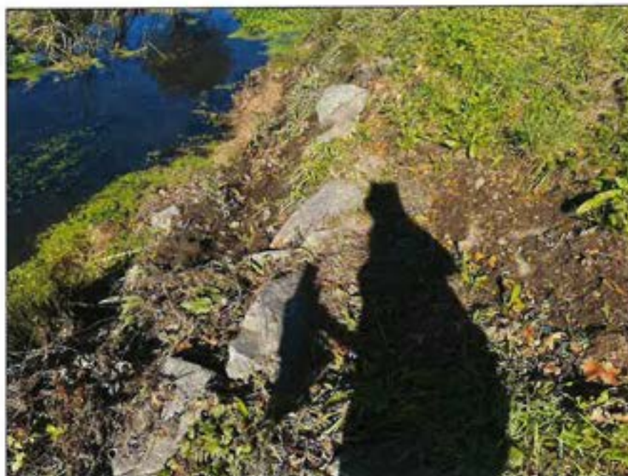
Photo No. 34.: Erosion on downstream slope near STA 54+00.
