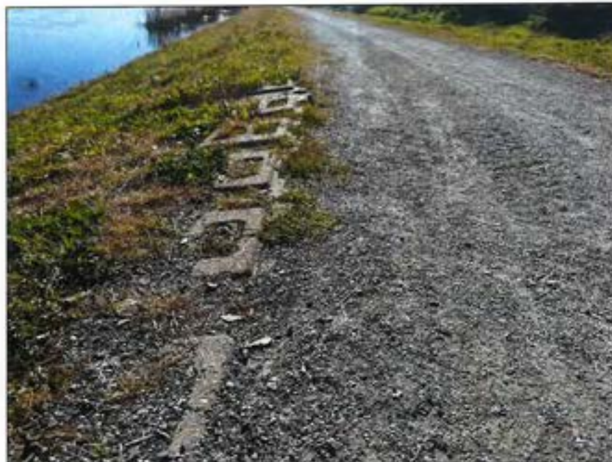
Photo No. 38.: Exposed ACBs slightly higher than the crest at the bend near STA 57+10.
