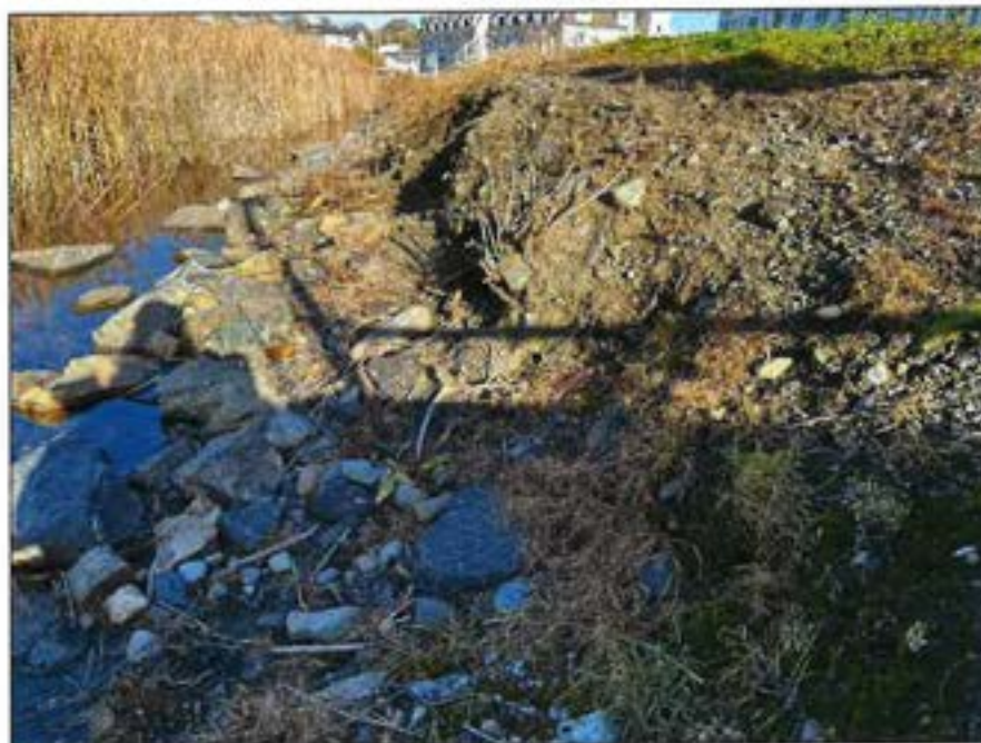
Photo No. 49.: Upstream slope to the left of the primary spillway. Note erosion.
