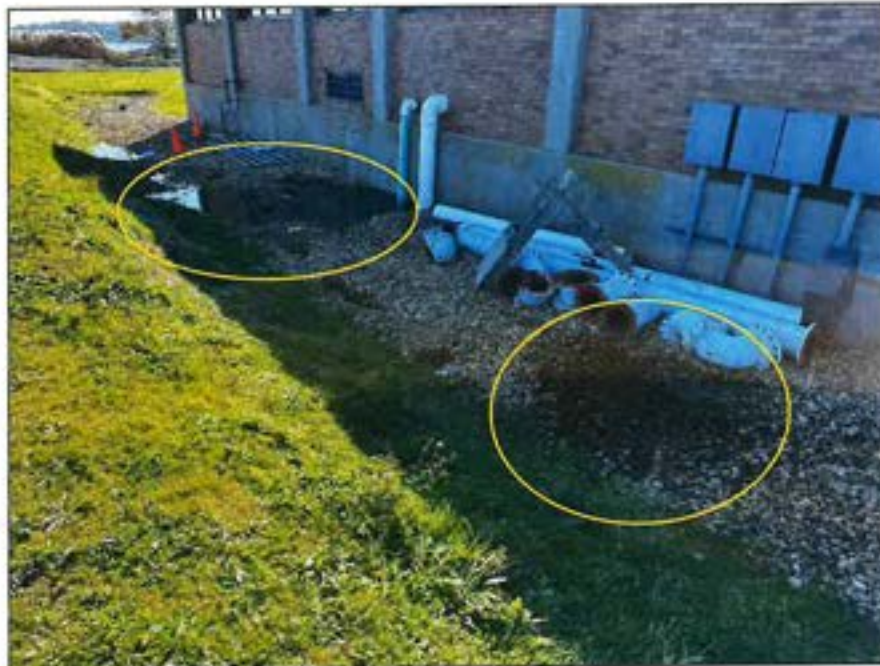
Photo No. 13.: Saturated area at downstream toe between STA 1+65 and 1+90.
