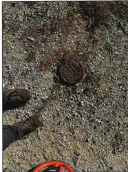
Photo No. 33.: Low level outlet valve cover.
