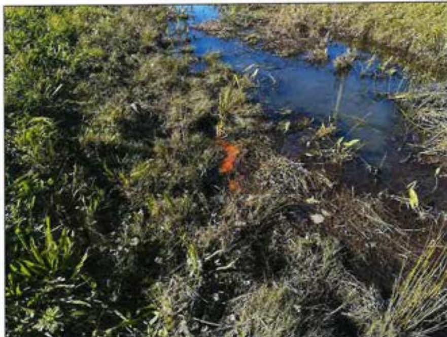
Photo No. 42.: Iron oxide staining at the tow of the downstream slope near STA 63+10.
