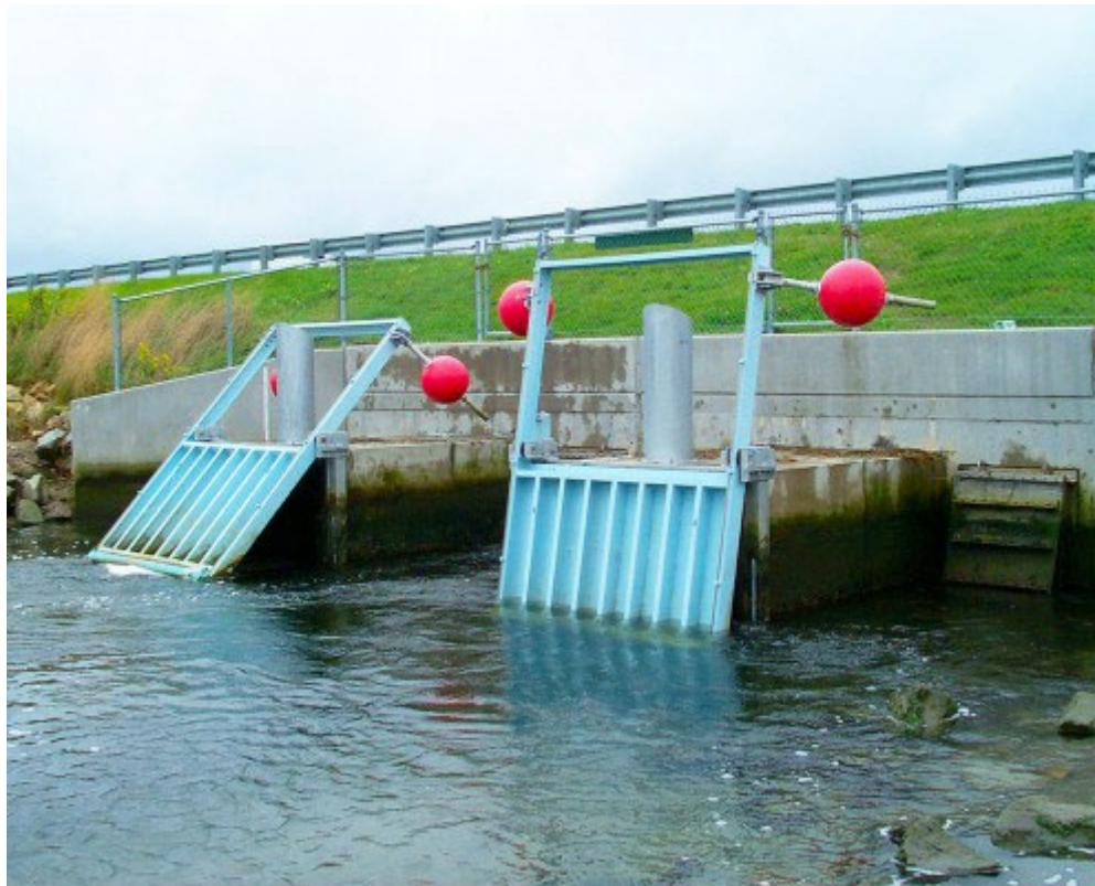
Figure 7: Tidal gate example ( https://watermanusa.com/products/large-custom-gates/self-regulating-tide-gates/ )
