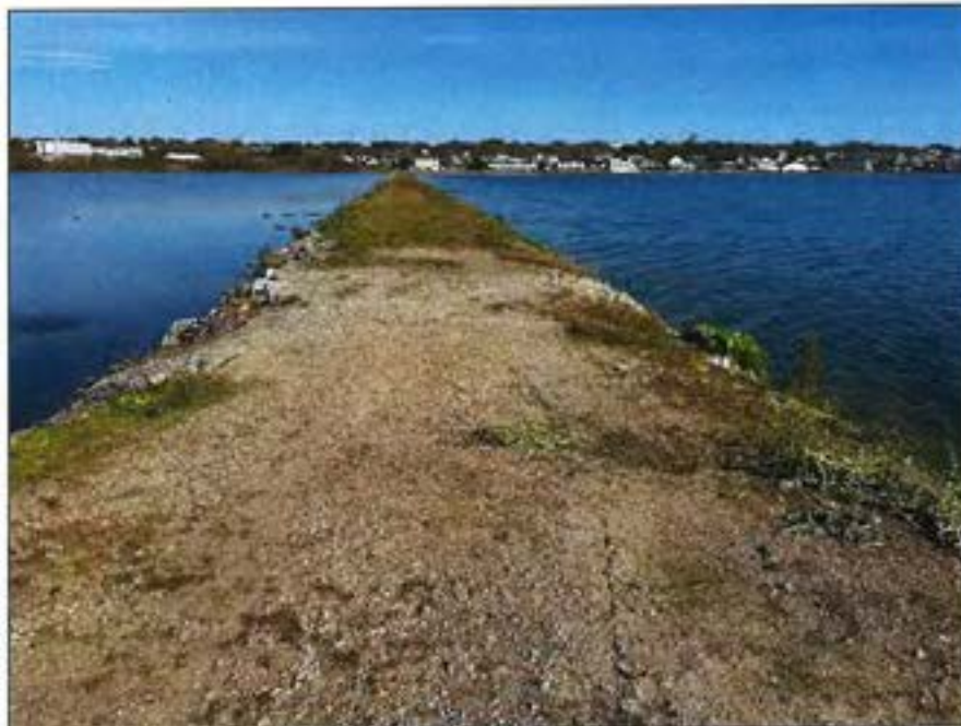
Photo No. 10.: Crest from the bend in the embankment near STA 10+50 looking left. Note bare soils at the bend.
