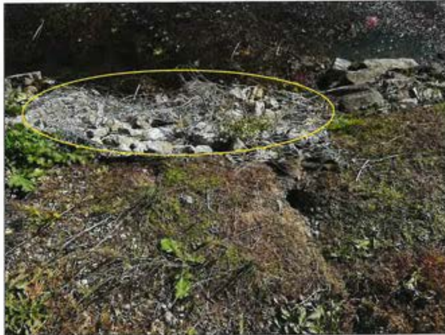
Photo No. 17.: Broken gabions near STA 16+50.
